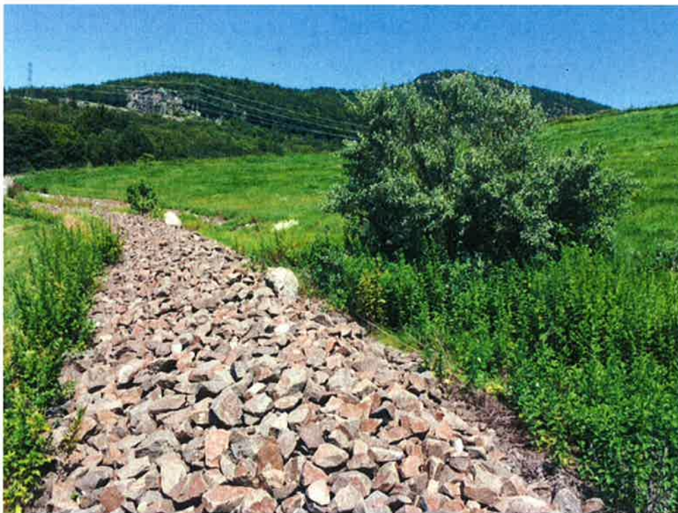
Photograph 14: Sapling growing adjacent to a side drainage channel to Downchute 1 on the southeastern portion of the Landfill (southeast to northwest).
