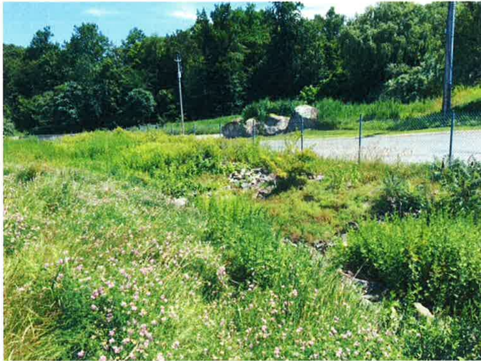
Photograph 7: More evidence of overgrown vegetation within the perimeter drainage structure along the northeastern edge of the Landfill (southwest to northeast).
