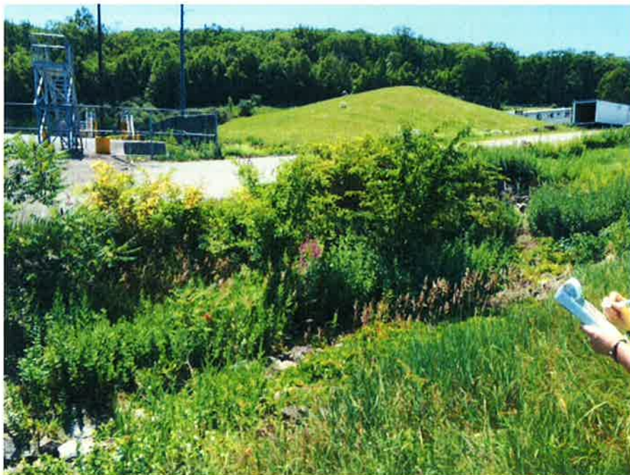
Photograph 6: Overgrown vegetation present within perimeter drainage structure along the northeastern edge of the Landfill (north to south).
