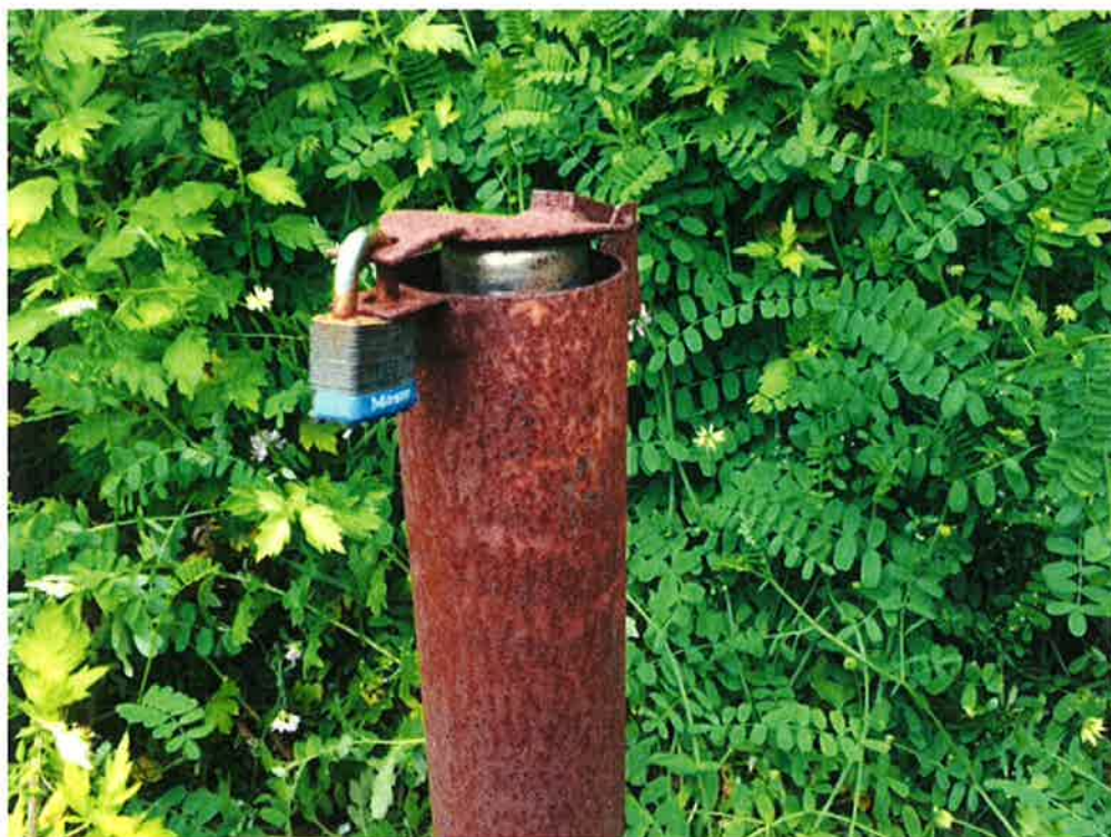
Photograph 1: Monitoring well 3-R locks, however, does not close properly and is open to the elements (east to west).
