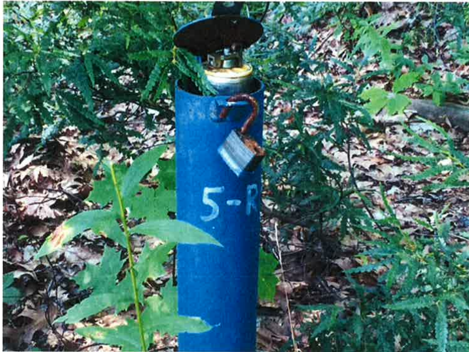
Photograph 15: Monitoring well 5-R cannot be properly closed and locked due to the PVC casing being longer than the steel protective casing (northwest to southeast).
