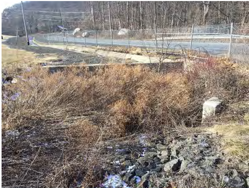
Photograph 5: Localized overgrown vegetation observed in drainage swale along the northern most portion of the Landfill.
