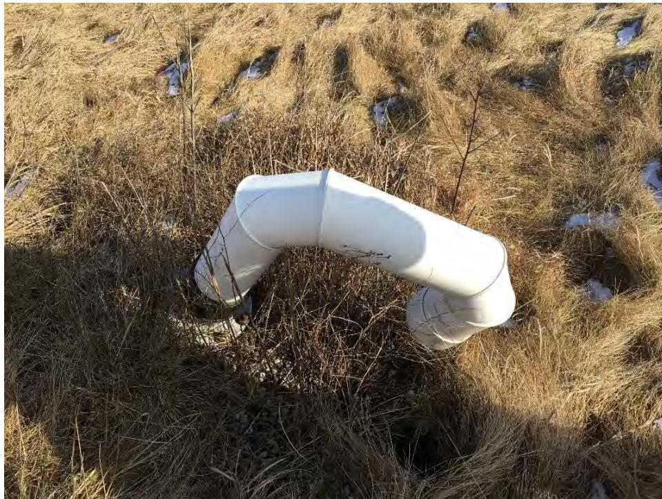
Photograph 16: Downed vent observed in mid-northern portion of the Landfill. STERLING propped vent up but could not fasten dislodged section of vent.
