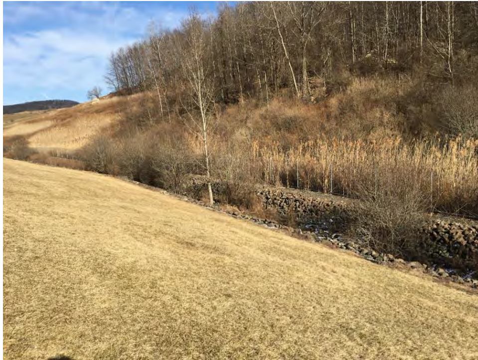
Photograph 13: Overgrown vegetation observed along the southeastern perimeter drainage ditch (southwest to northeast).
