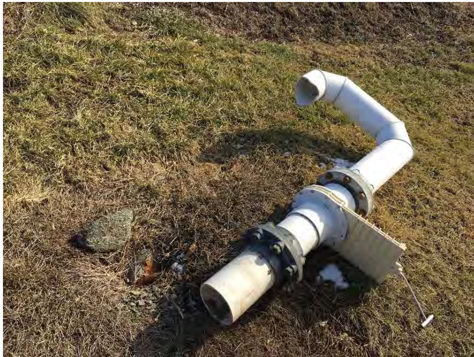
Photograph 12: Downed vent observed on the southwestern sideslope of the Landfill.
