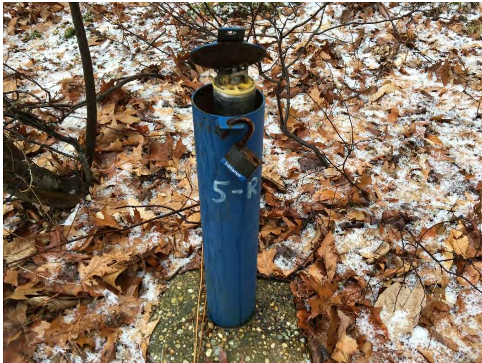
Photograph 20: Monitoring well 5-R (utilized for depth to water measurements only) is not able to close and lock (west to east).
