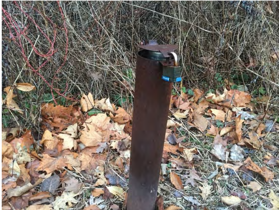
Photograph 25: Monitoring well 3-R (utilized for depth to water measurements only) is locked, NOTE: top flap of protective casing is not tight with the locking hasp (southeast to northwest).
