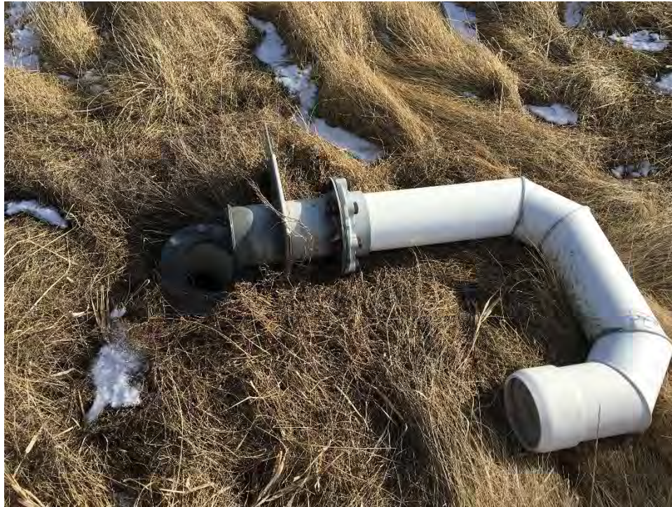
Photograph 17: Downed vent observed in central portion of Landfill.
