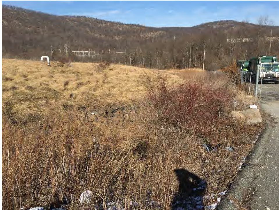
Photograph 3: Patch of overgrown vegetation observed in perimeter drainage ditch along the eastern portion of the Landfill (south to north).
