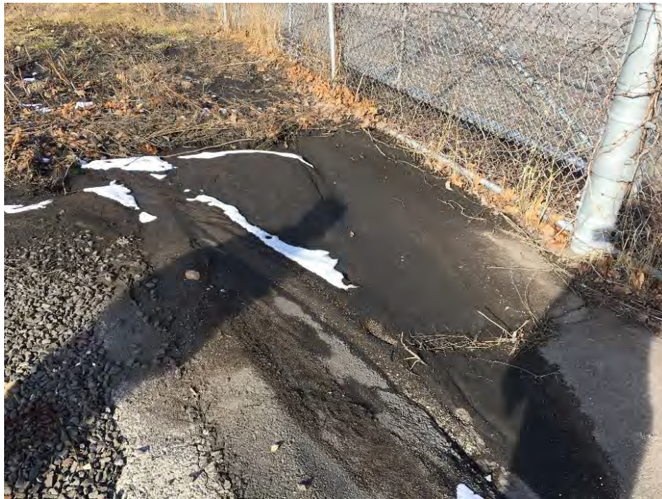
Photograph 4: Build-up of sediment observed near drainage swale along the northernmost portion of the Landfill (south to north).
