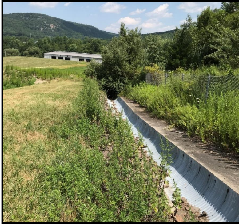
Photograph 3: View of northeast perimeter drainage system, looking northeast.
