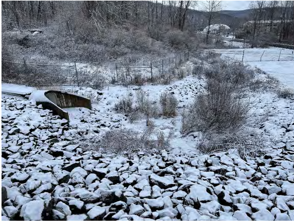
Photograph 21: View of overgrown vegetation in drainage feature along the southern perimeter of the Landfill, looking south.
