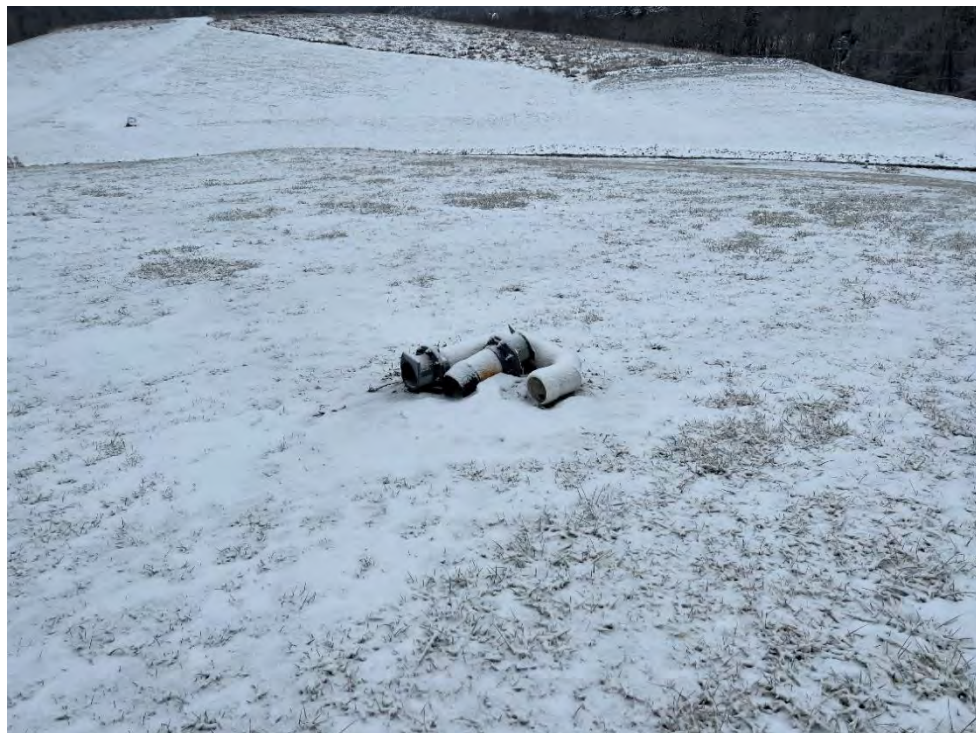
Photograph 6: View of damaged gas vent near the midwestern perimeter of the Landfill, looking south.
