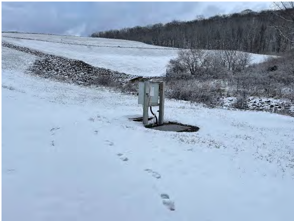
Photograph 20: View of Lift Station W-20 in the southwestern portion of the Landfill, looking east.
