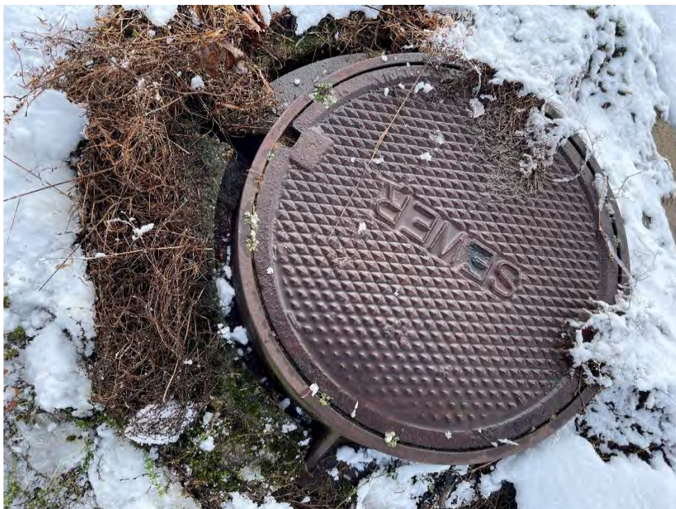
Photograph 2: View of damaged upper portion of the concrete drainage vault (MH E-6) near the northern perimeter of the Landfill, looking southeast.
