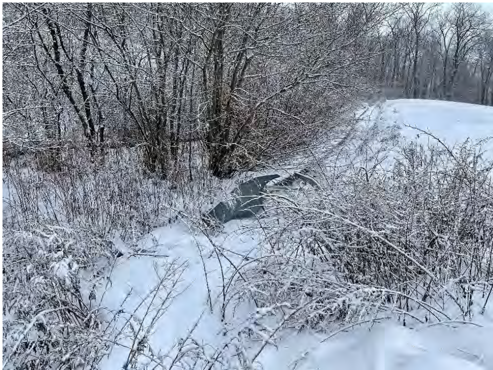
Photograph 16: View of debris build-up in drainage swale along the northeastern perimeter of the Landfill, looking south-southwest.
