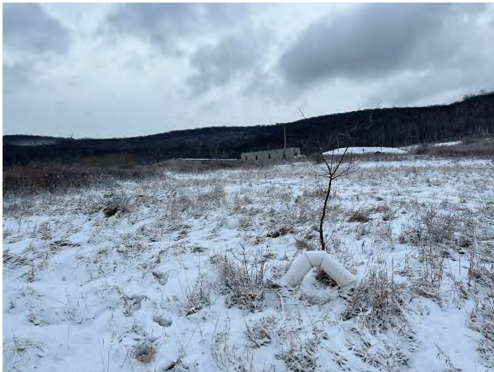
Photograph 4: View of leaning gas vent in the north central portion of the Landfill, looking southeast.
