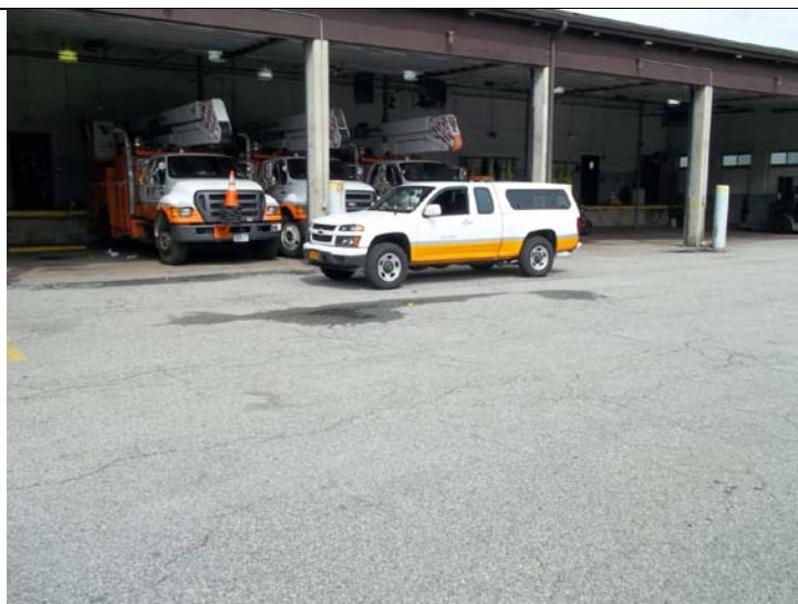
Depressions and cracks in asphalt cover
