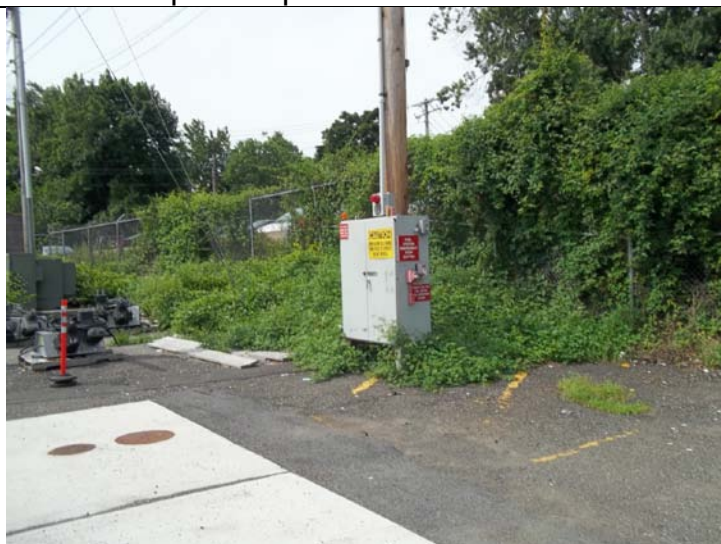
Vegetation along edge of asphalt cap
