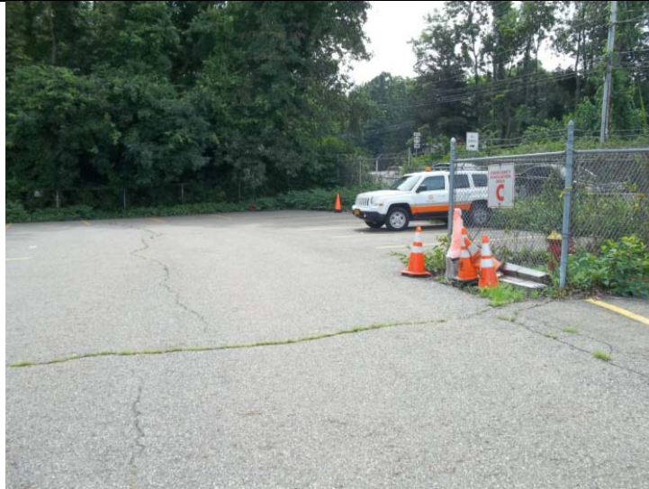
Cracks in asphalt cover
