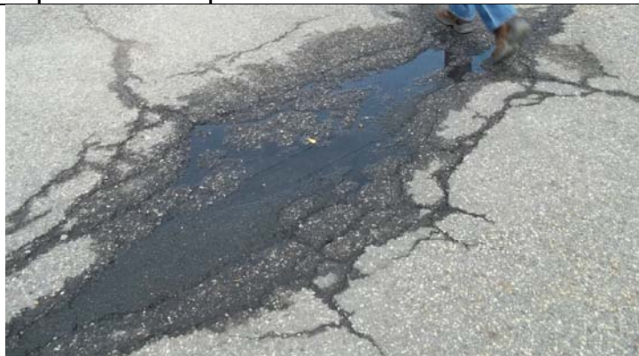
Depression in asphalt cover, soil not exposed
