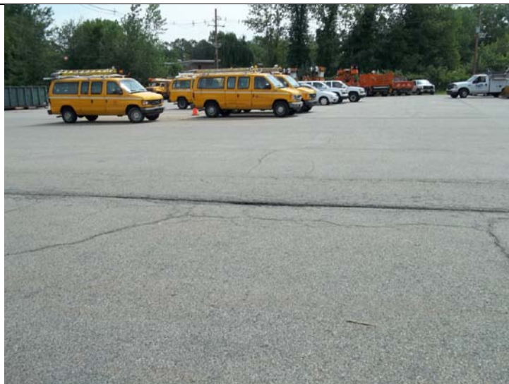
Cracks in asphalt cap
