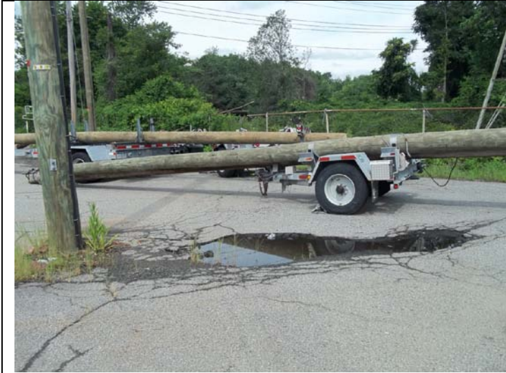
Depression in asphalt cover
