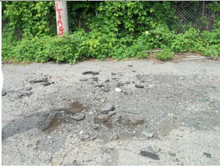
Scattered asphalt and dirt, asphalt cap does not appear to be impacted
