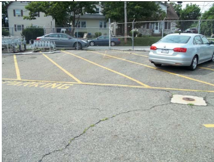
Cracks in asphalt cover, monitoring, fencing intact
