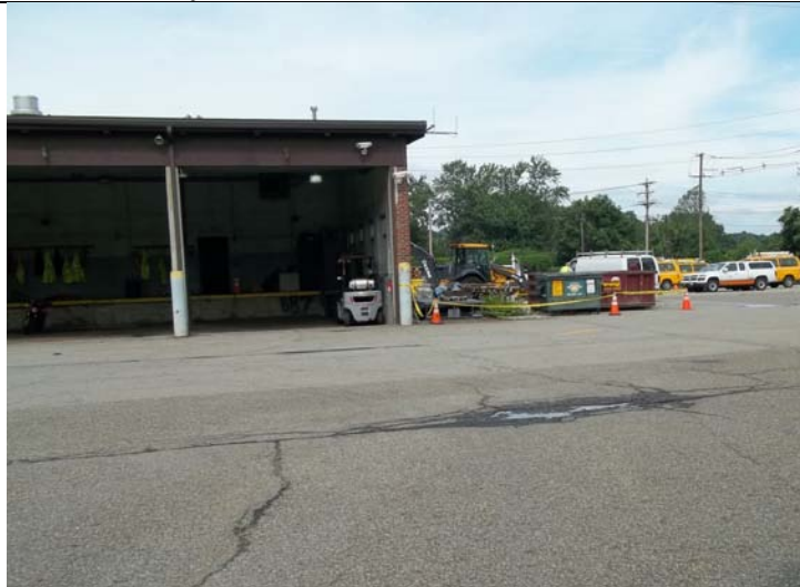
Depression in asphalt cover
