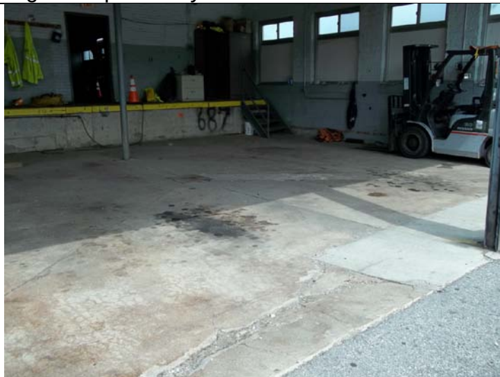
Cracks in garage floor
