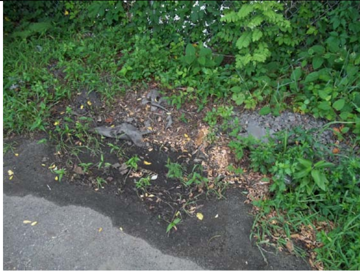
Edge of asphalt may need maintenance
