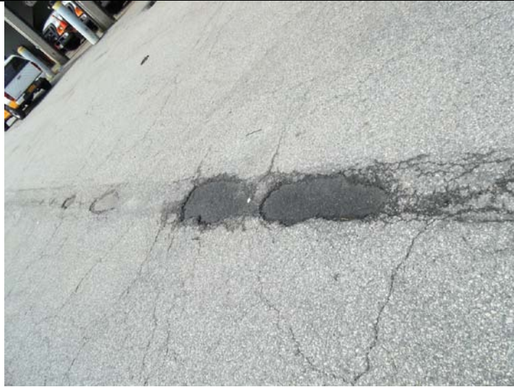
Depression in asphalt cover, soil not exposed
