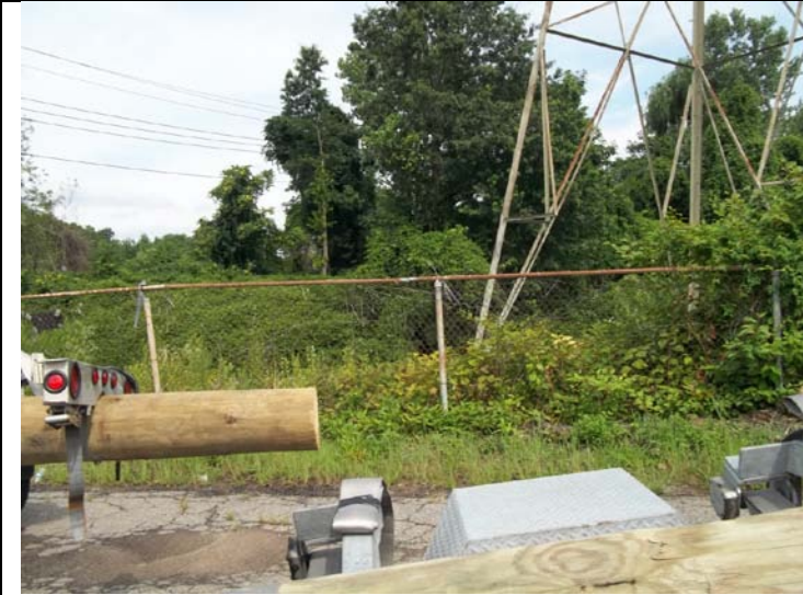
Fence appears to be loose at top railing
