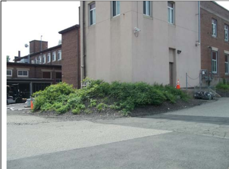
Oiled stone chips along building, some chips are falling off the mound
