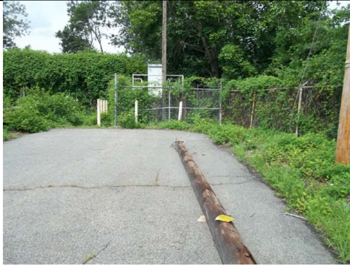
Cracks in asphalt cap, wood pole
