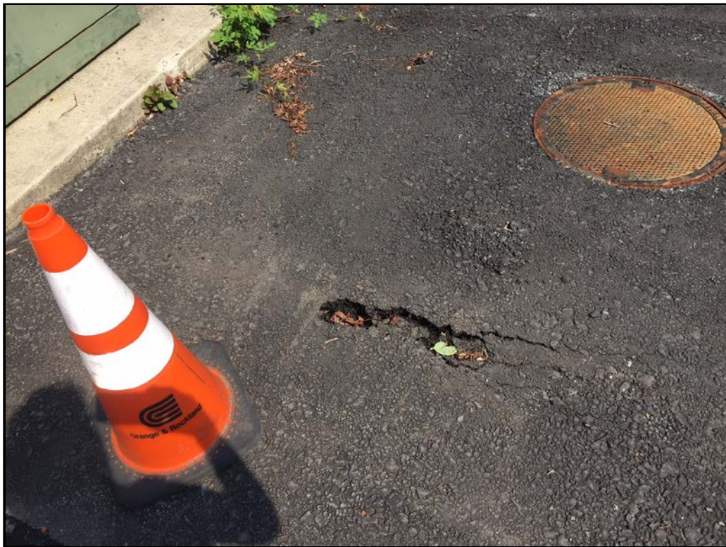
PHOTOGRAPH 8 Depression/Crack in Pavement Patch for New Emergency Generator
