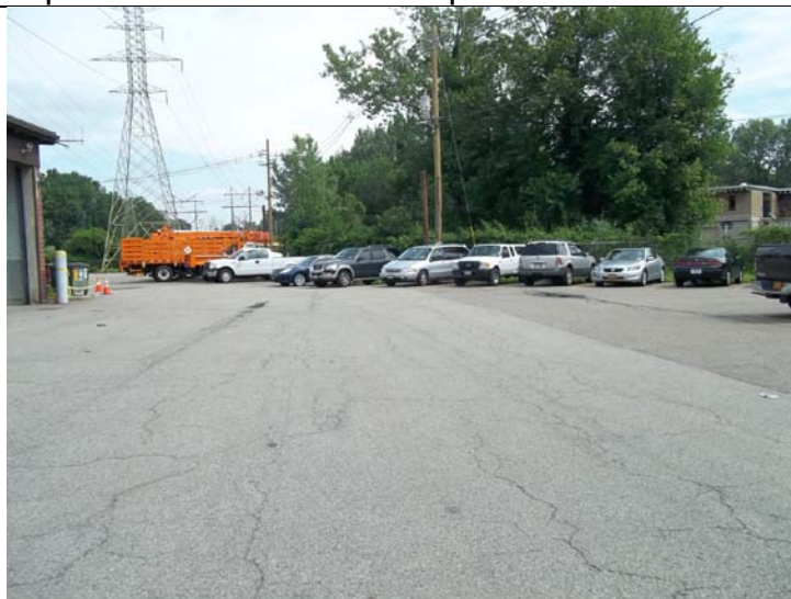
Depressions and cracks in asphalt cover
