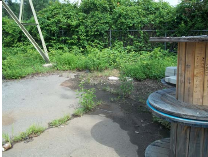
Cracks in asphalt cover, soil may be washed onto asphalt cover
