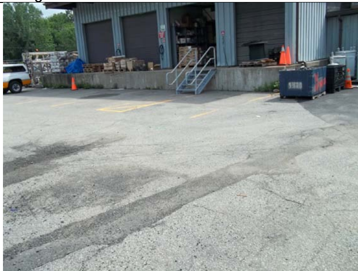
Trench pre-dates the July 2012 Site Management Plan, depression in asphalt cap
