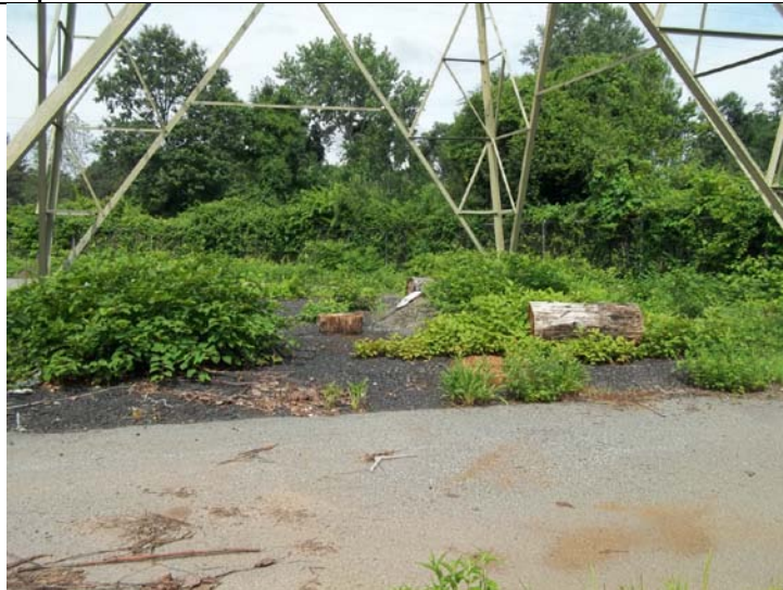
Oiled stone chips under towers
