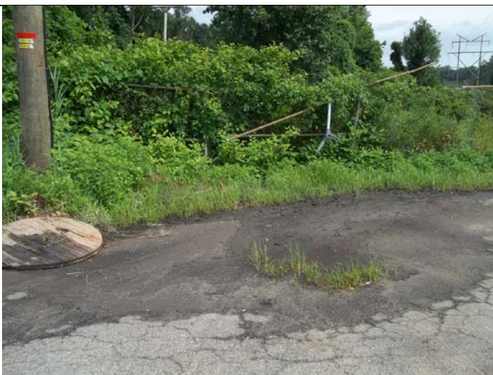
Soil appears to be washing onto asphalt cap, wood debris
