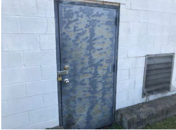
Photo 1: Door to the area containing the pump and treat system was secured with a padlock.
