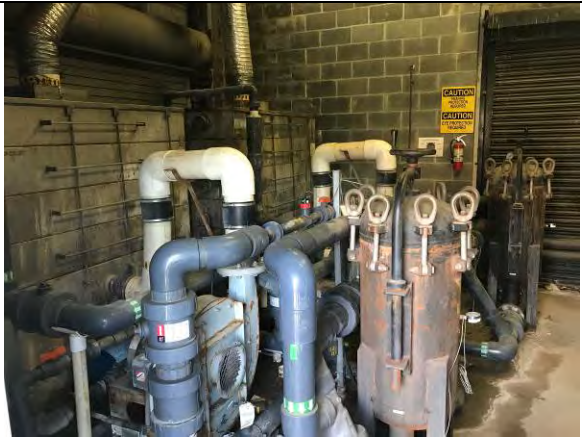
Photo 10: The pump and treat system.
