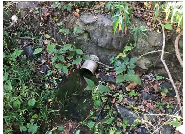
Photo 4: The effluent pipe for the pump and treat system.
