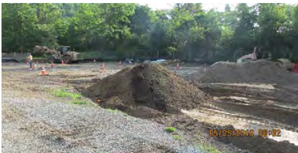
05 25 16 sparge wells and site
