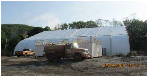
05 25 16 sparge wells and site
