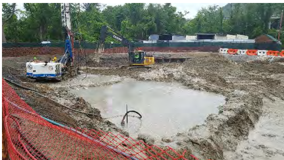
05 25 17 - Rain Water Area D
