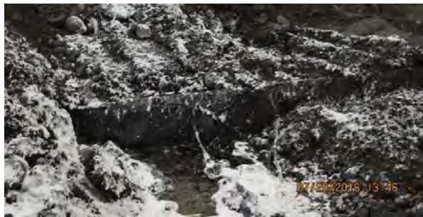
07 29 16 Bottom of holding tank Area D
