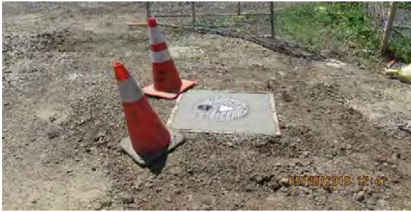
05 20 16 water line and sparge wells
