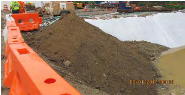
08 01 16 Fresh Backfill covering erosion
