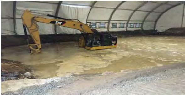
08 01 16 Area B2 Flooding
