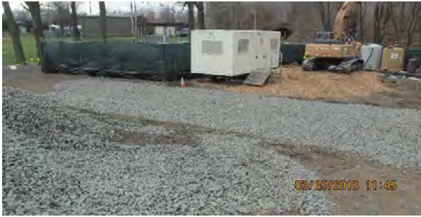
03 25 16 WTP and site
