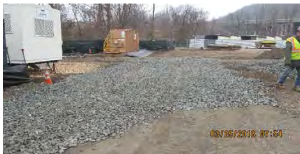
03 25 16 WTP and site
