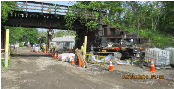
05 20 16 water line and sparge wells
