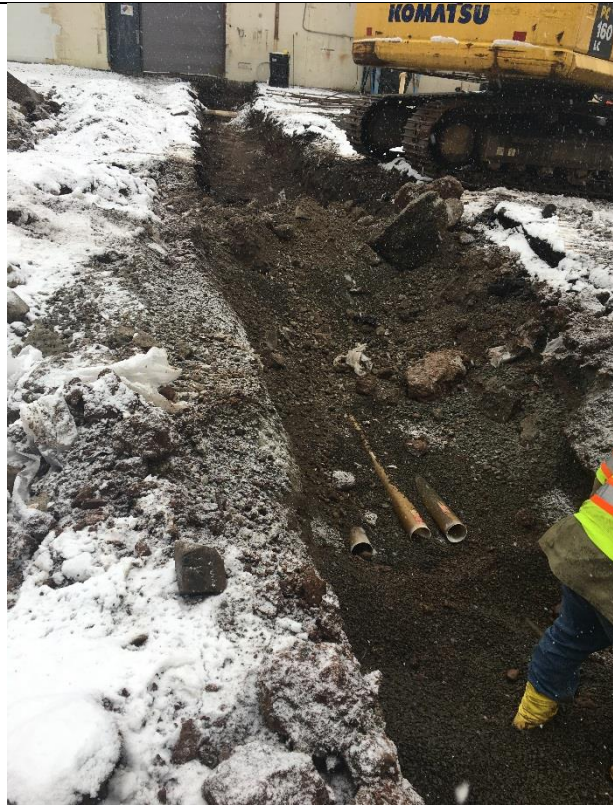
Photograph: 7 | Exposed pipes in pipe run
