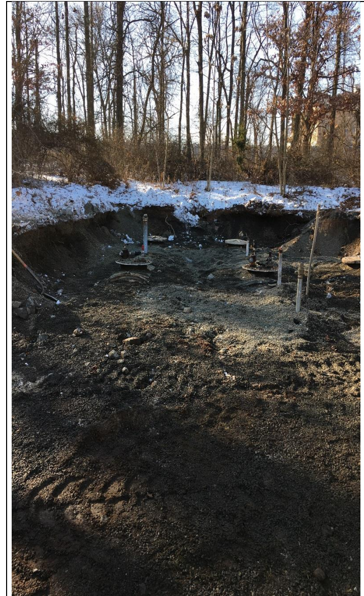
Photograph: 2 | Exposed fill ports
