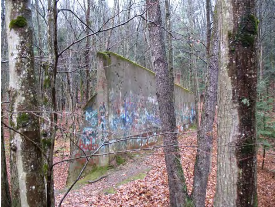
Photograph 3: View facing east of backstop wall showing bullet markings (4 December 2008) Oneonta Rifle Range (old) (RRNY000021)
