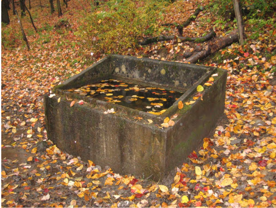
Photograph 1: 4' by 4' by 3' concrete reservoir near the targets (16 October 2008) Hoosick Falls Range (new) (RRNY000012)
