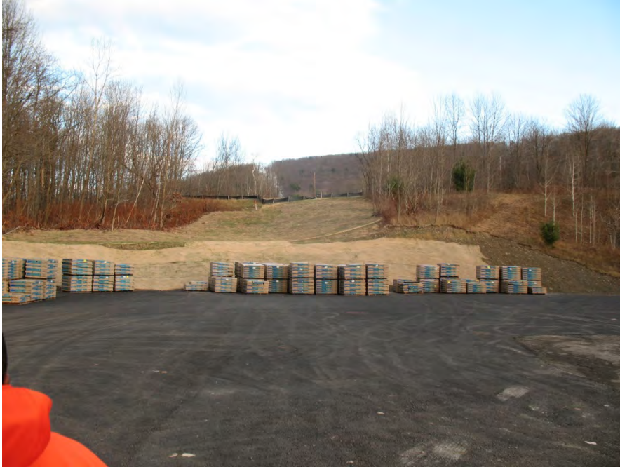
Photograph 3: View of northern portion of C & L Property recently reconstructed (3 December 2008) Binghamton Rifle Range (new) (RRNY000002)
