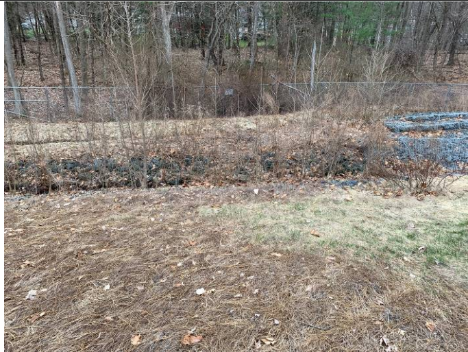
Photo 11: Looking south. View of small trees growing in the southern drainage channel.
