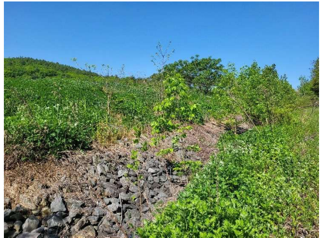
Photo #10: View of the northern drainage channel, which contains some overgrowth present, facing west.
