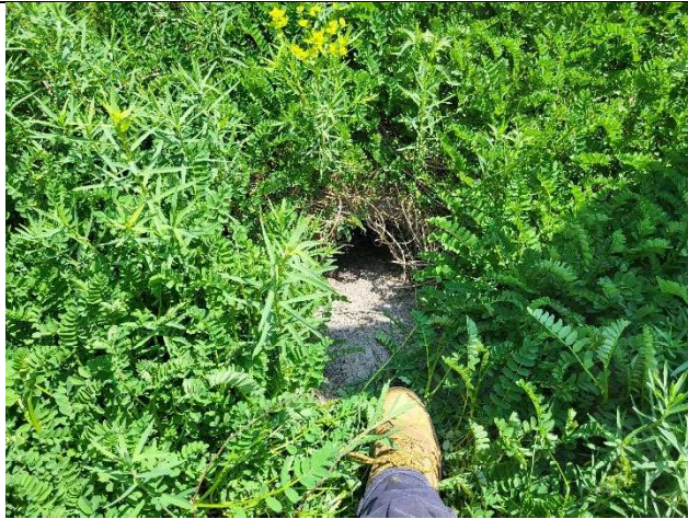
Photo #7: View of a rodent hole observed along the northern end of the landfill, facing west.
