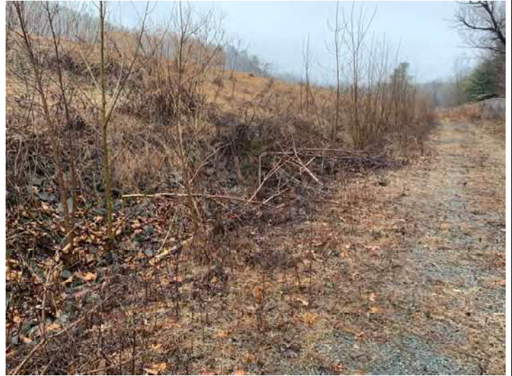
Photo 6: Looking west. View of overgrown trees in northern rip rap channel.
