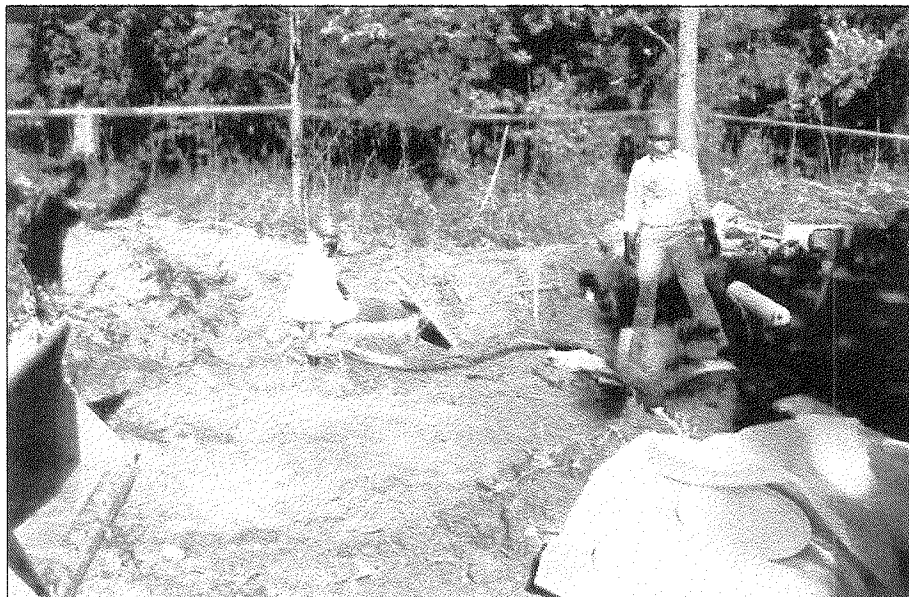
Photo 1. Tank with pump setup. (9-23-97)
