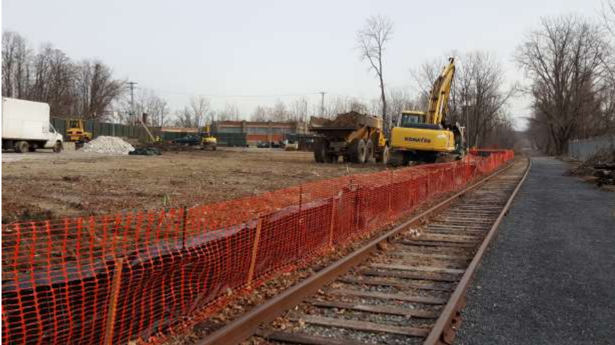
Photograph 4: Silt fencing was installed and maintained at the hydraulically downgradient perimeter of the site and offsite excavation area for erosion control. Construction fencing was also installed to secure site access. Photograph facing east along south property line.
