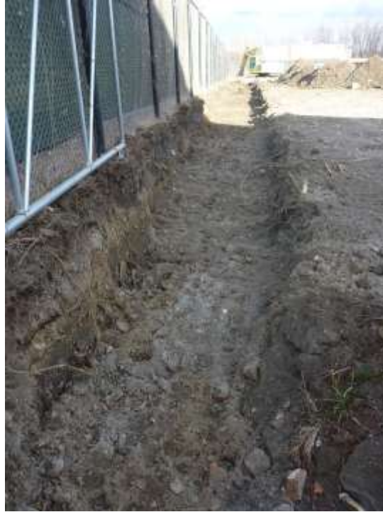
Photograph 14: Approximately two (2) feet of soil located north of the Millens property line and south of the site's fence line was excavated by Ulster Excavating and placed in the soil placement area and covered.
