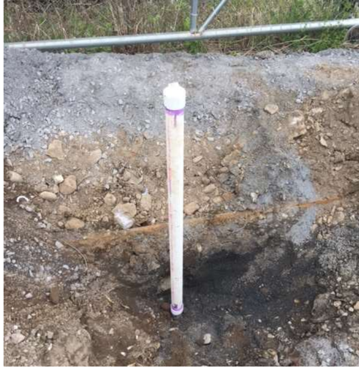
Photograph 25: Ulster Excavating located the remainder of the below grade portion of MW-10, repaired the associated well casing and installed a new protective casing on April 29, 2016.
