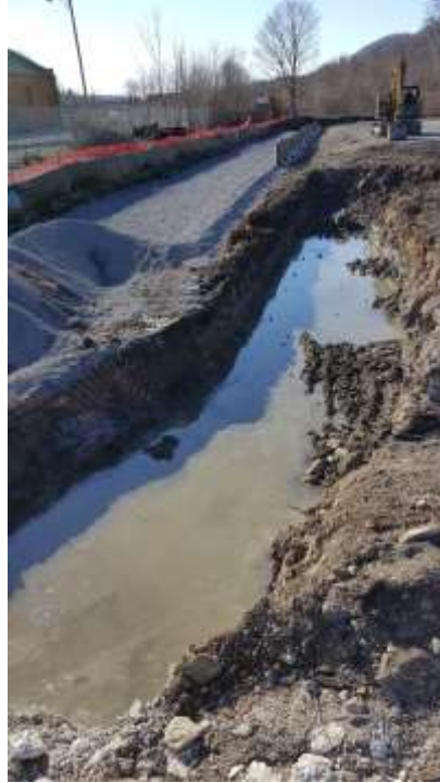
Photograph 16: Stained soil shown in Photograph 15 was excavated and placed in the soil placement area and covered. Photograph facing west.
