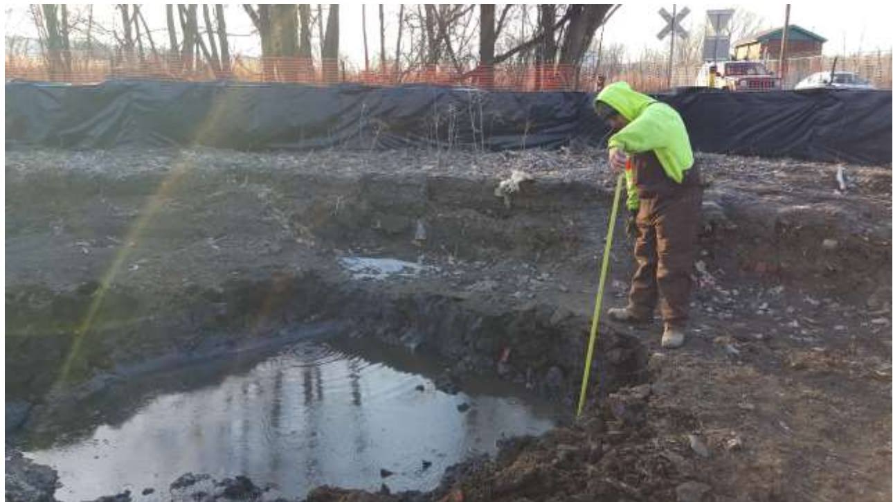
Photograph 17: Ulster Excavating excavated additional soil from the offsite area east of North Street and removed all impacted soil. Excavated soil was placed within the soil placement area and covered.
