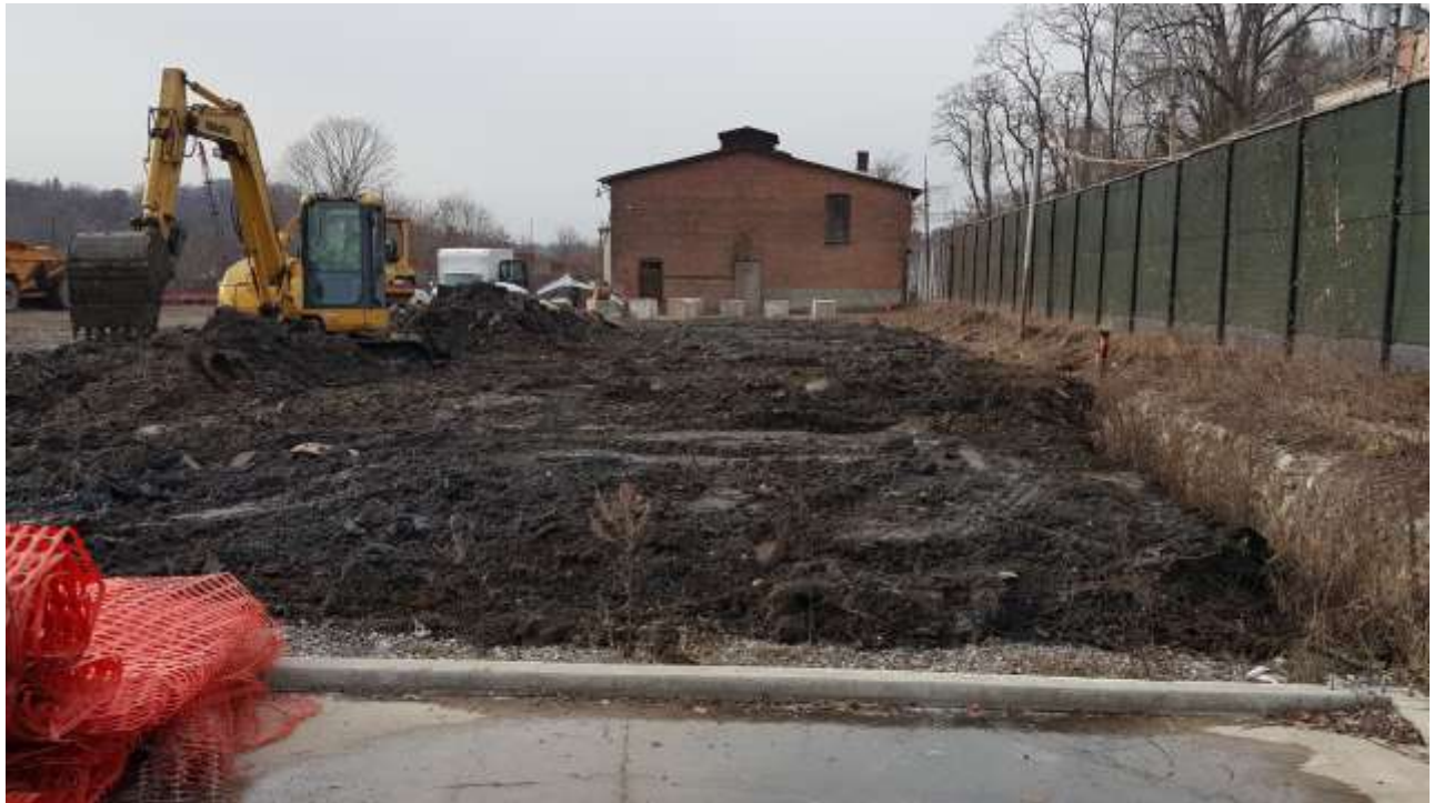
Photograph 7: Onsite and offsite soils excavated by Ulster Excavating were placed in the designated soil placement area. Soil stockpiles were temporary and were graded before the end of each work day.
