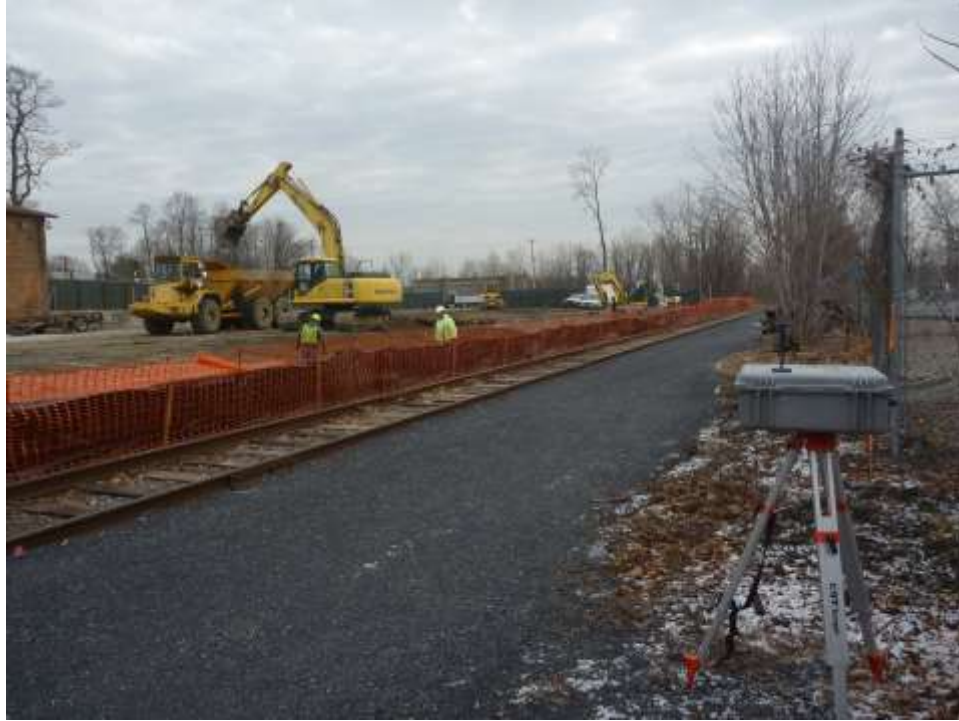
Photograph 10: Perimeter community air monitoring was conducted during ground-intrusive activities and during moving and placement of impacted soil.
