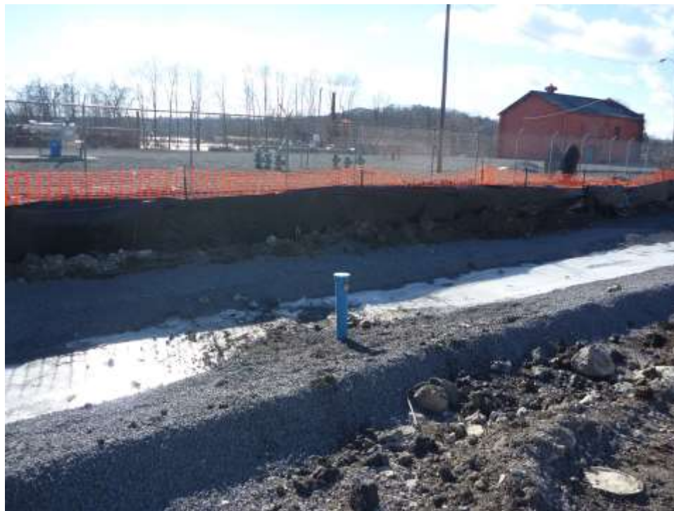
Photograph 26: The well casing associated with MW-14 was replaced by ADT to accommodate new site grades. The top of the PVC well casing was cut and resurveyed.
