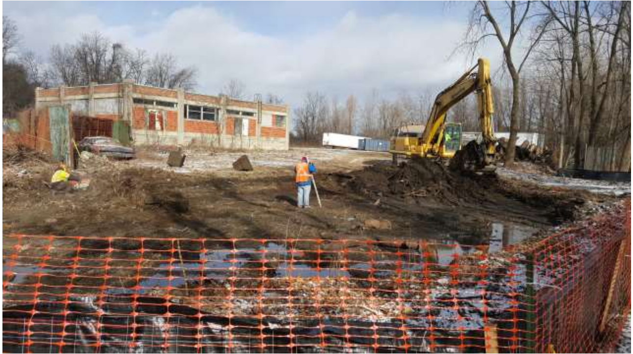
Photograph 6: Ulster Excavating excavated impacted soil from the offsite area east of North Street and confirmatory sampling was conducted to verify the removal of impacted soil.
