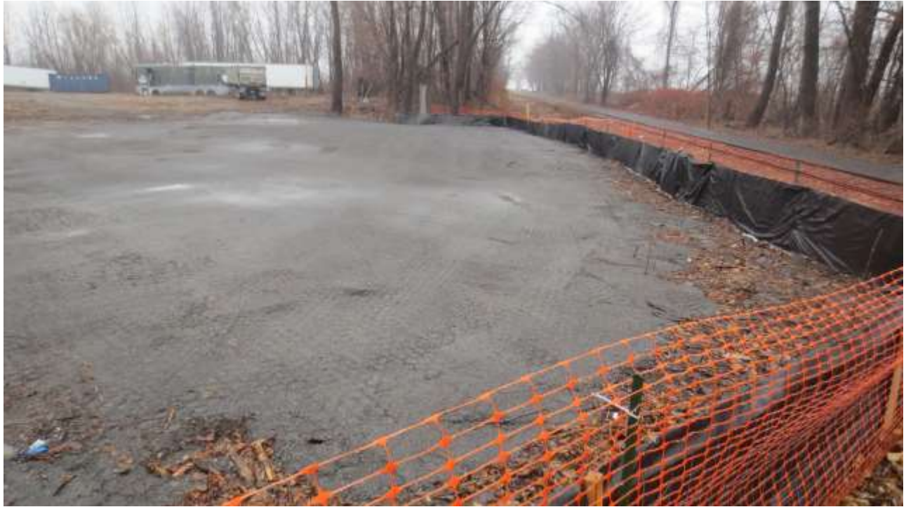
Photograph 27: Imported stone product was placed within the offsite excavation area located east of North Street. No demarcation layer was installed in the offsite excavation area because end-point sampling indicated that impacted soil was removed.
