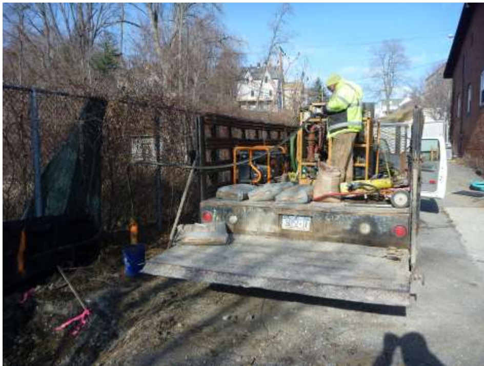
Photograph 11: Monitoring wells MW-1, MW-2, and MW-7R were decommissioned by ADT in accordance with the Interim Remedial Measures (IRM) Work Plan dated November 18, 2015 and Commissioner's Policy-43 (CP-43). Monitoring well MW-2 shown above.
