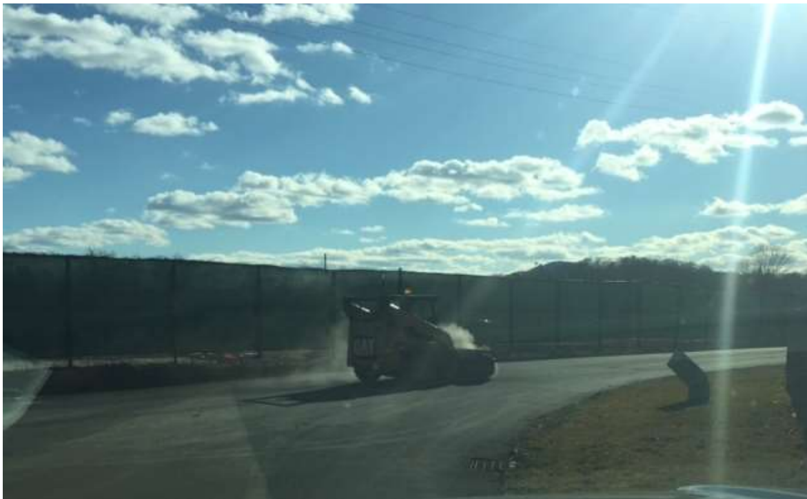
Photograph 9: Public roadways abutting the site were swept by Ulster Excavating, as necessary, to mitigate potential nuisance dust conditions.
