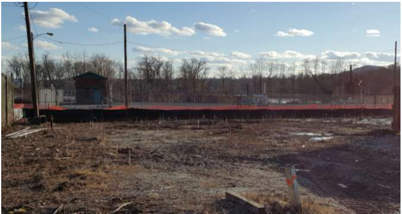
Photograph 3: Oxygen Release Compound Advanced® (ORC) injection points were marked with wood stakes during site preparation activities.
