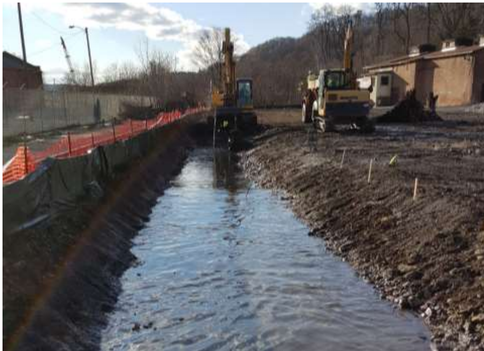
Photograph 5: Site soil was excavated by Ulster Excavating & Trucking, Inc. (Ulster Excavating) to achieve intended site grades and for the construction of a stormwater control ditch along southern property boundary, shown above. Photograph facing west.
