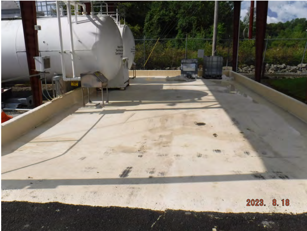
LOADING / UNLOADING AREA FOR 6,000-GALLON AST
