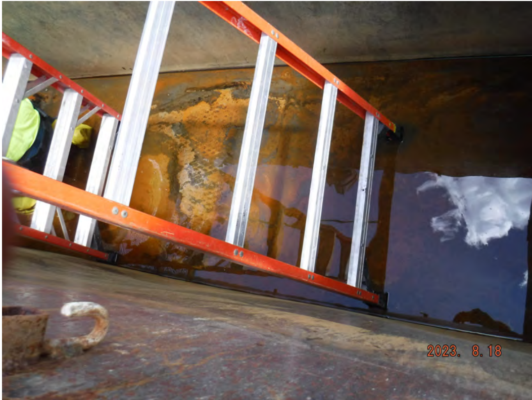
INTERIOR OF PCB SOAKING TANK
