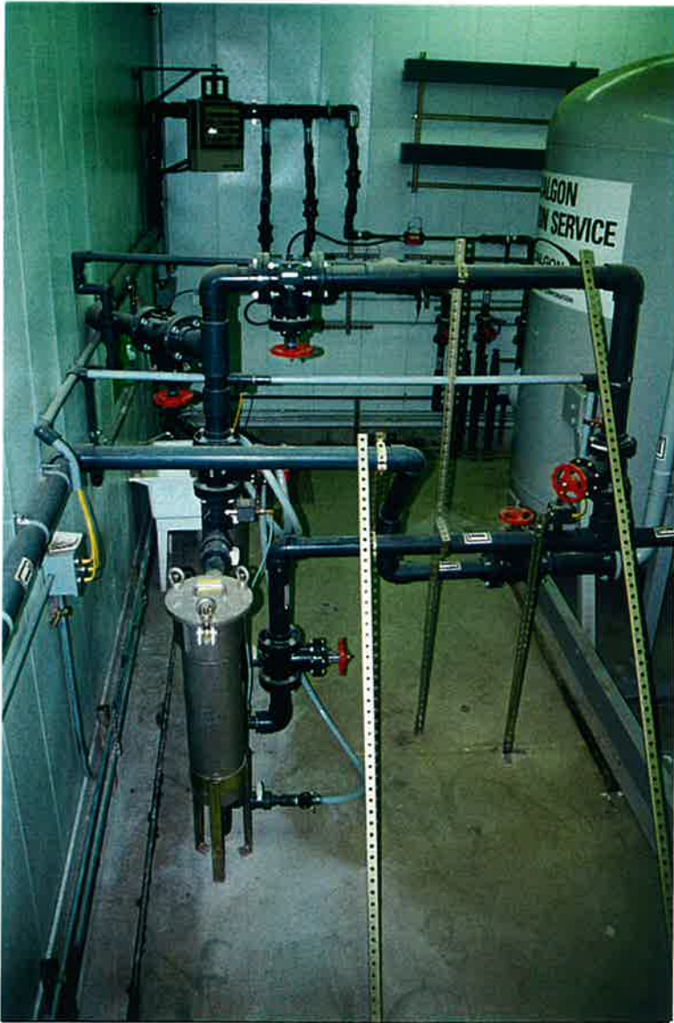
Internal Piping, Supports, Bag Filters and Carbon Units.
