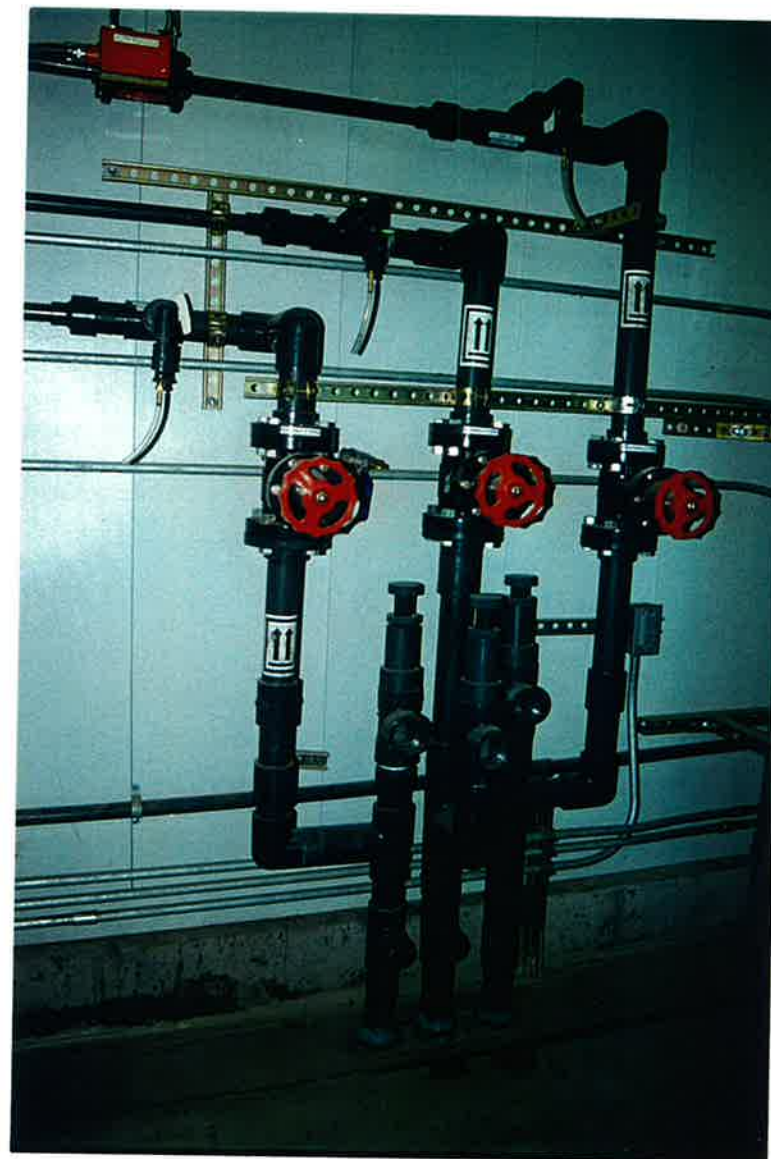
EW-1, EW-2, EW-3 piping at West Wall.
