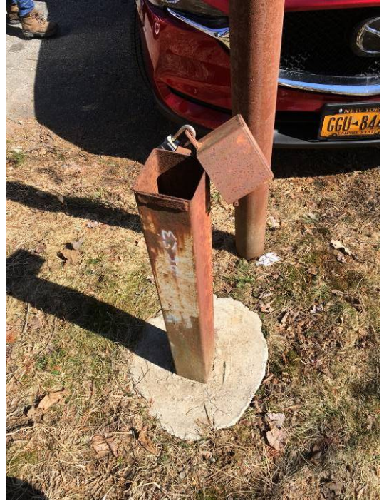
Photo 2: Photo of BVWSA-MW-U9 with damaged casing cap
