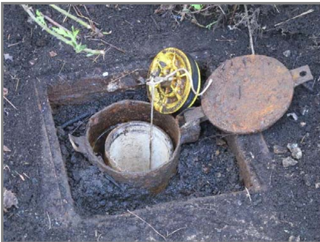
Closeup of MW-4B. This shallow roadbox type installation has a loose fitting cover. Mulch, dirt and fill holds it down.
