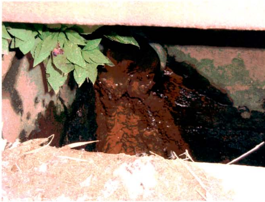
Figure 7. Sample 8 was a solid sample of iron floc accumulating in a pipe conveying groundwater from the landfill site to the catch-basin on Taylor Lane.
