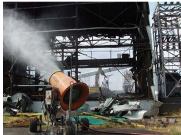
FIGURE 9-1: Dust Control. Minimizing dust during demolition is a critical element of the Building 52 project to protect the surrounding community and environment.
