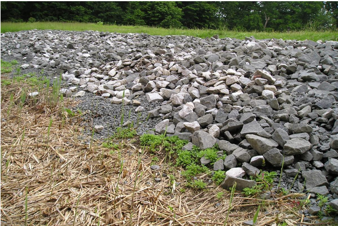
Photo 24: West slope erosion area repair (looking east)
