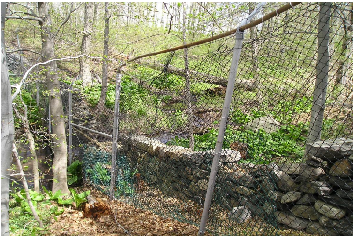
Photo 16: Fallen tree removed off fence and repairs were made (near stream inlet – northeast of landfill cap)
