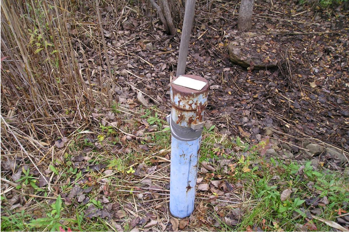
Photo 7: Well PC-1 (with broken key in lock)
