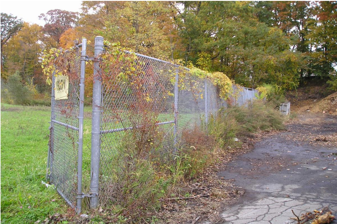
Photo 12: South fence damage (looking east)
