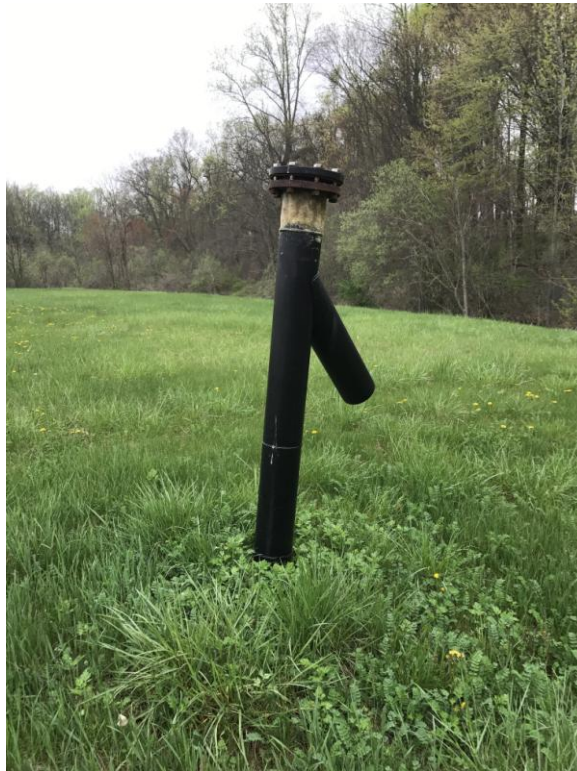
Photo 2: Vent V-2 (repair patch shown)
