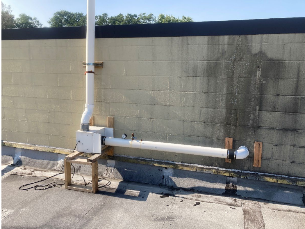
Photograph 4: View of in-line fan on the side of HomeSense.
