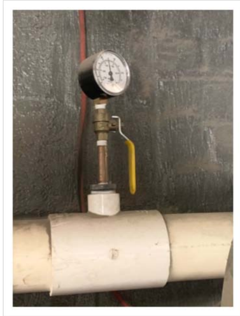
6. Vacuum Gauge of the SVE System in the Repair Shop Area
