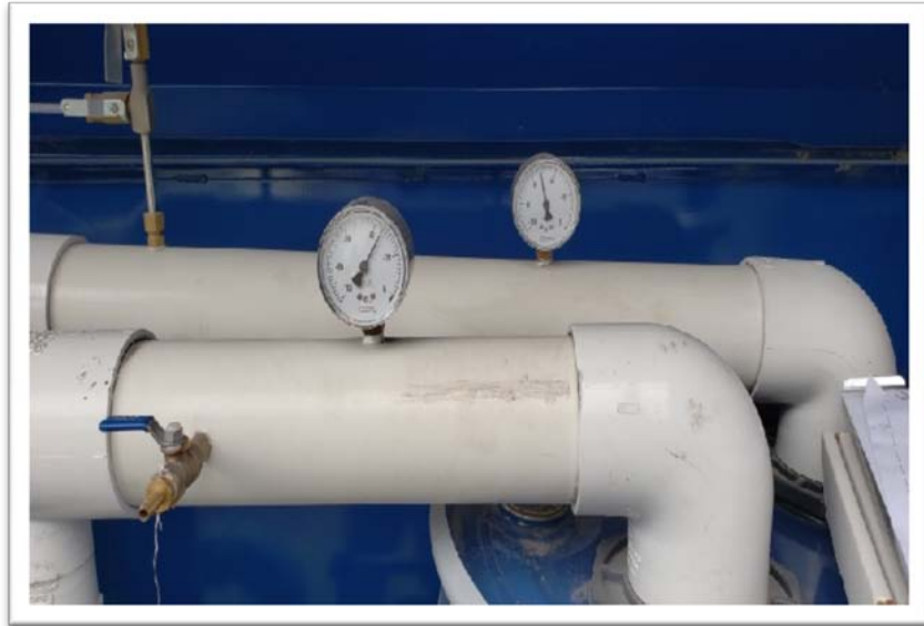
7. Vacuum Gauges of the SVE System Unit
