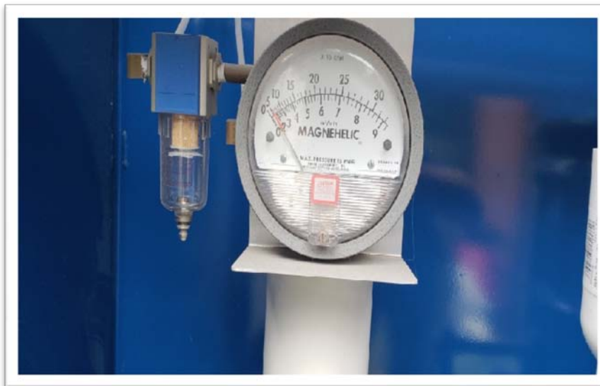
4. CFM Reading at the SVE System Unit
