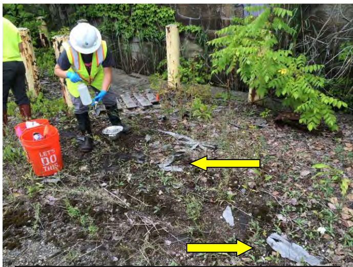
Photo 2. Bulk Galbestos on the ground surface
