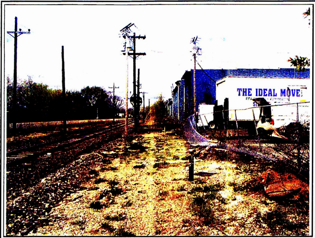
Photograph 3. Dislodged chain link fence at south end of paved parking area between Buildings 14 and 16.
