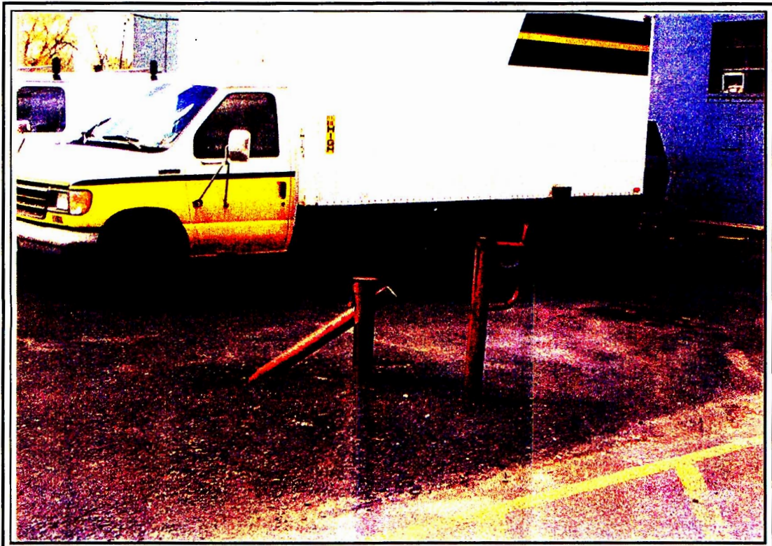
Photograph 2. Damaged protective bollard for MW-1 located at northwestern corner of the paved parking area between Buildings 14 and 16.
