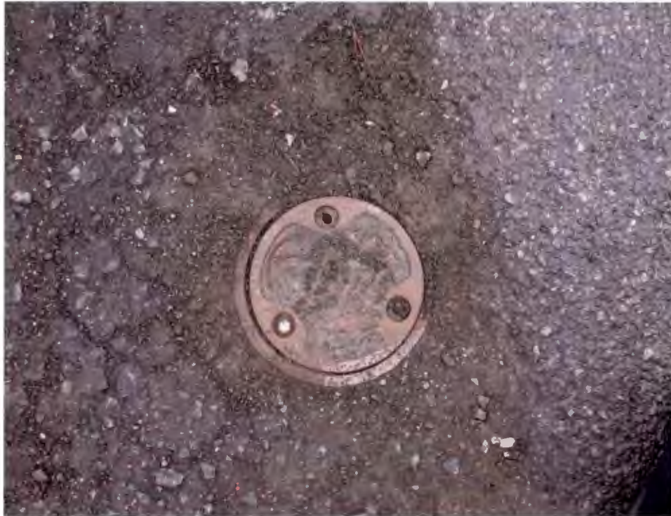
Photograph 1. Flush-mount Monitoring Well MW-1 located at northwestern corner of the paved parking area between Buildings #14 and #16.
