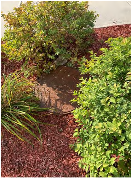
Picture 5: Sewer manhole lines did not lead within scope.
