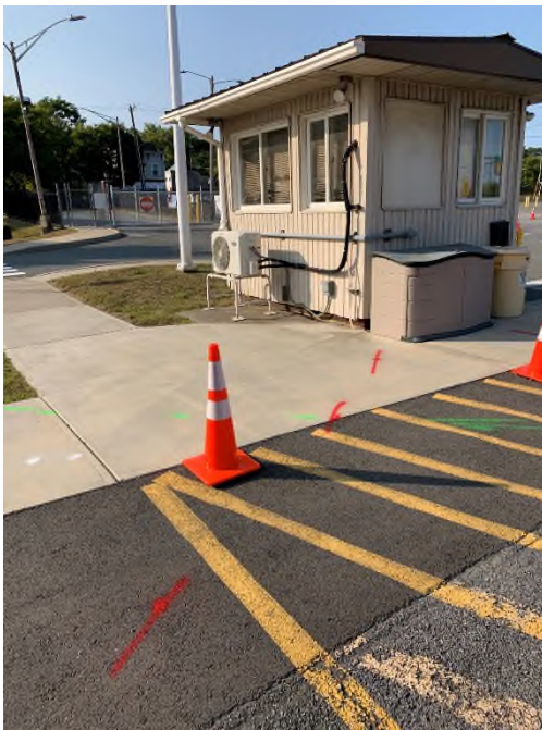
Picture 6: Electrical conduit from building going into security post.
