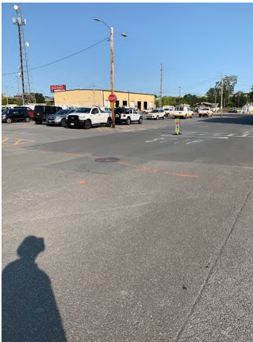
Picture 2: Communications manhole. Conduits going into the building and straight out the other way. Conduits going to the building looked as if they were cut.
