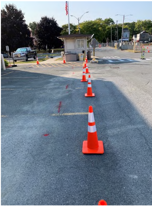
Picture 1: Electrical conduit coming out of security post.
