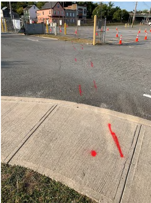
Picture 8: Electrical from guard post going towards electrical gate.
