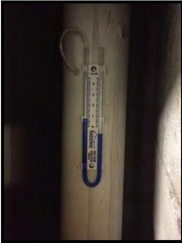
Photo 2: System manometer mounted to system pipe in basement
