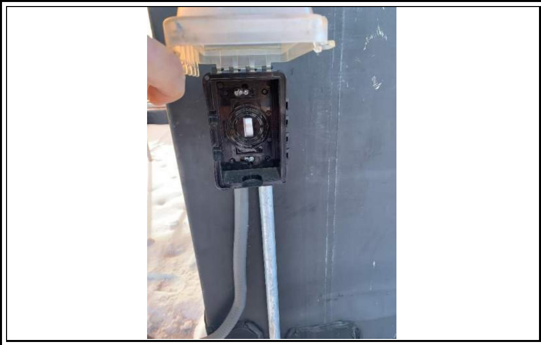
Photo 25: Electrical switch for fan at 140 State Street (12/14/22).
