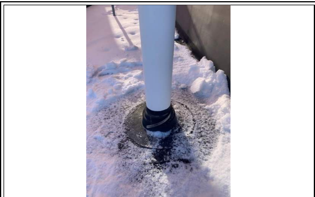
Photo 24: Close-up view of roof penetration/seal for SSDS exhaust stack at 140 State Street (12/14/22).
