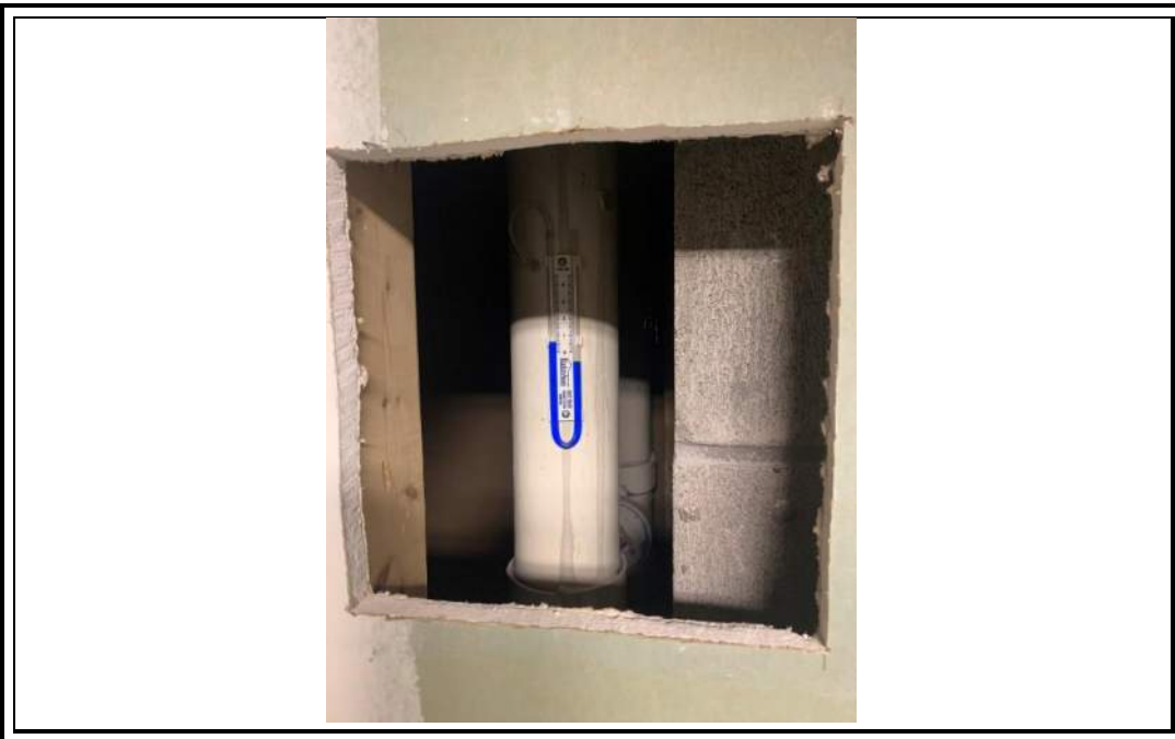
Photo 26: View of manometer and vertical riser pipe for SSDS at 140 State Street (access via basement level) (12/14/22).
