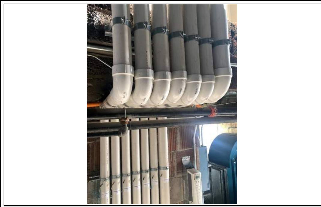
Photo 3: Riser piping for individual subsystems at 144 State Street (12/14/22).
