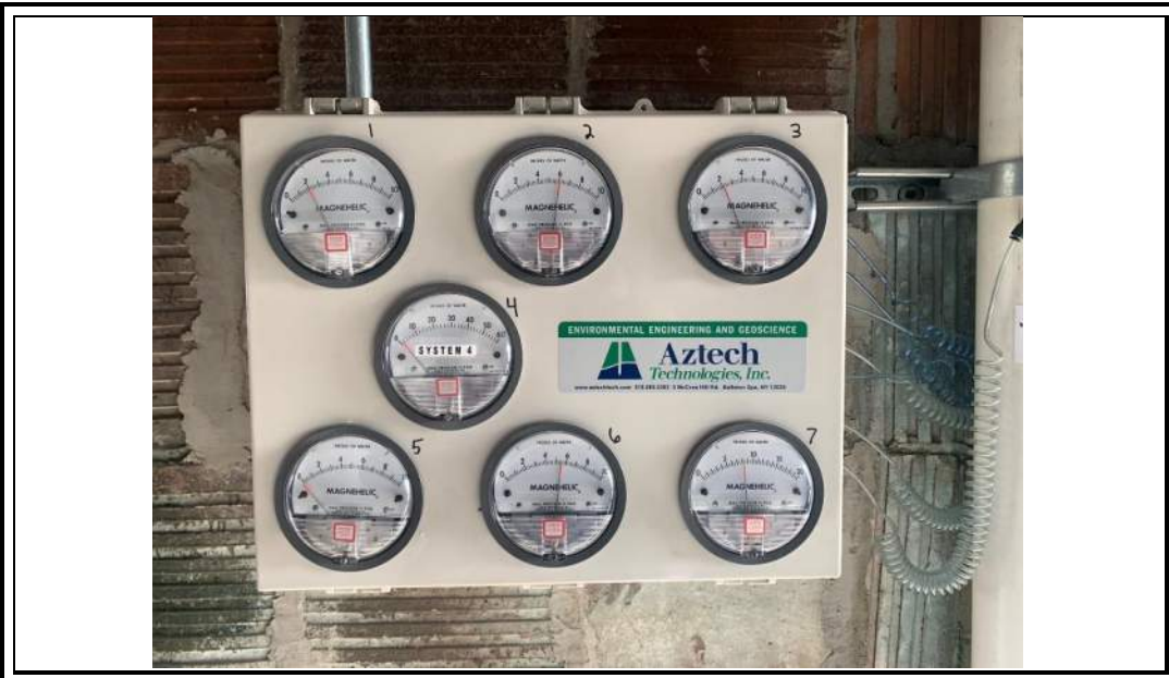
Photo 2: Close-up view of manometer panel for individual subsystems and tubing associated with the magnehelic manometers (12/14/22).
