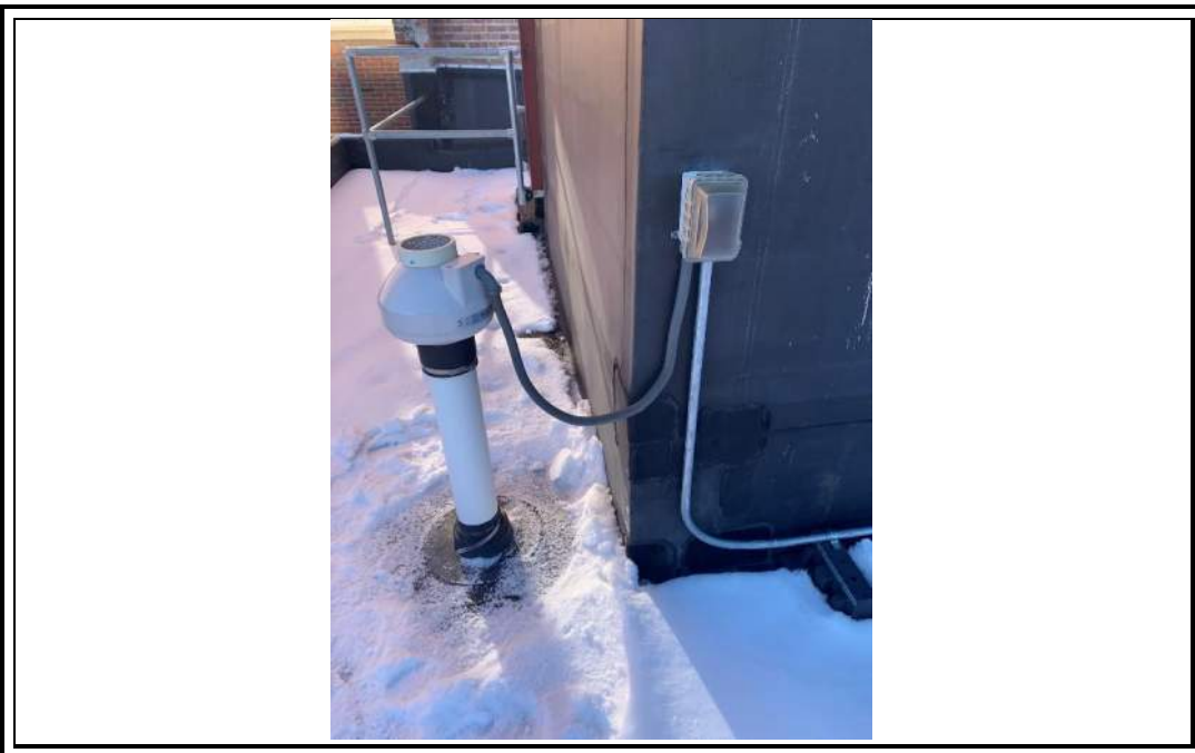
Photo 22: Roof of 140 State Street building; exhaust stack, fan and switch for SSDS (12/14/22).
