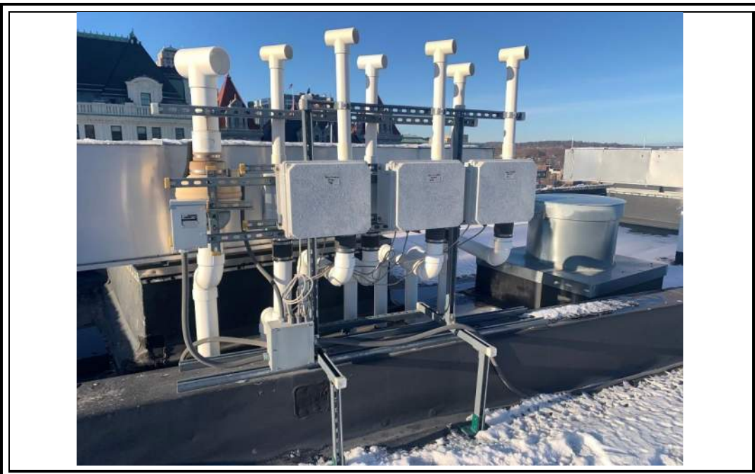
Photo 6: Roof-mounted fan units for individual sub-systems at 144 State Street (12/14/22).
