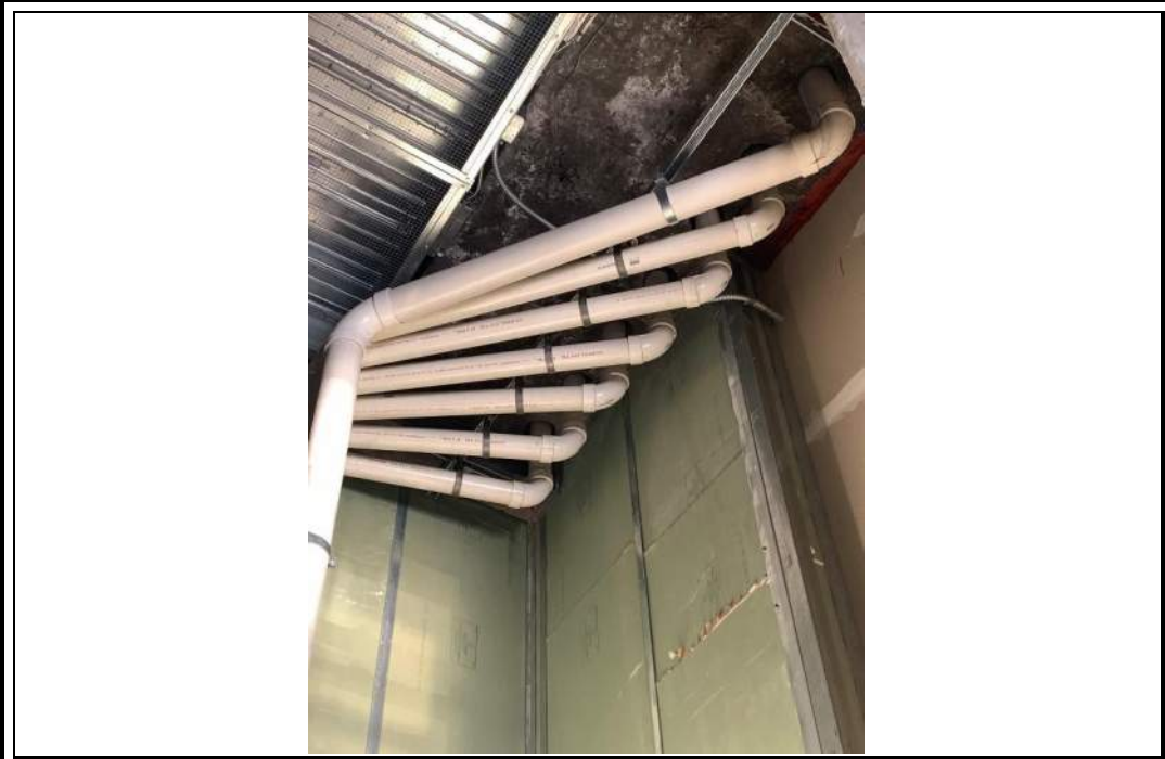
Photo 5: Riser piping for individual subsystems extending through the building roof at 144 State Street (12/14/22).
