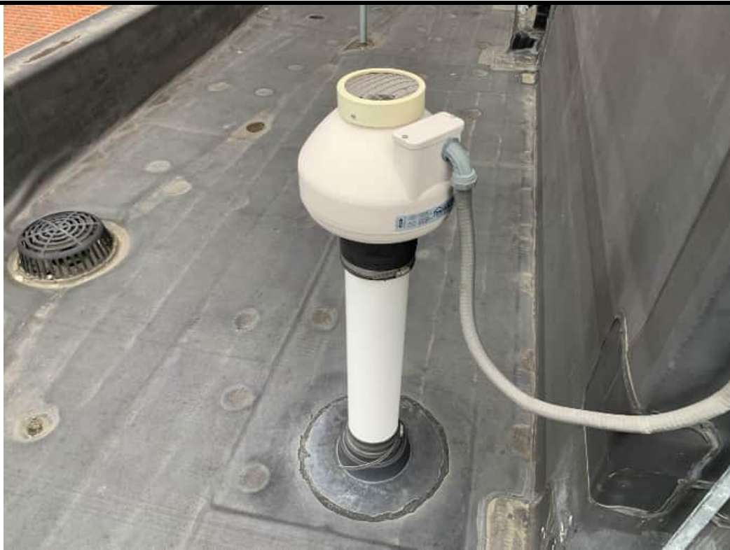
Photograph 17. Roof of 140 State Street building; exhaust stack, fan and switch for SSDS (12/20/24).
