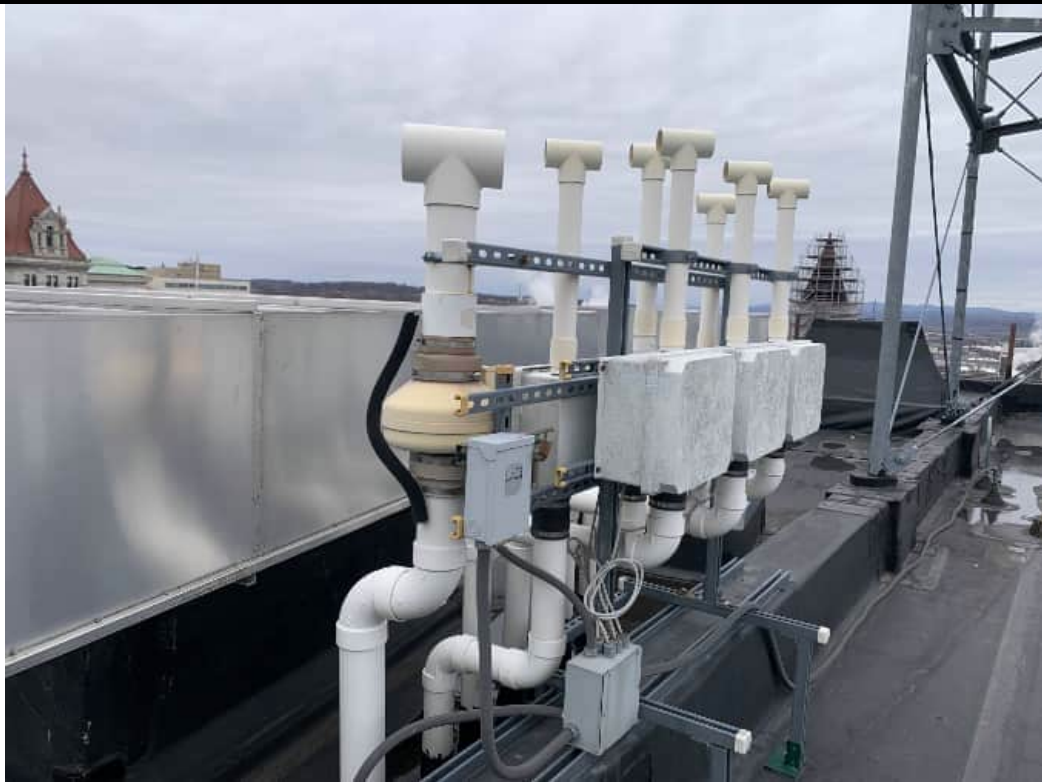
Photograph 6. Fan units for subsystems at 144 State Street (12/20/24).
