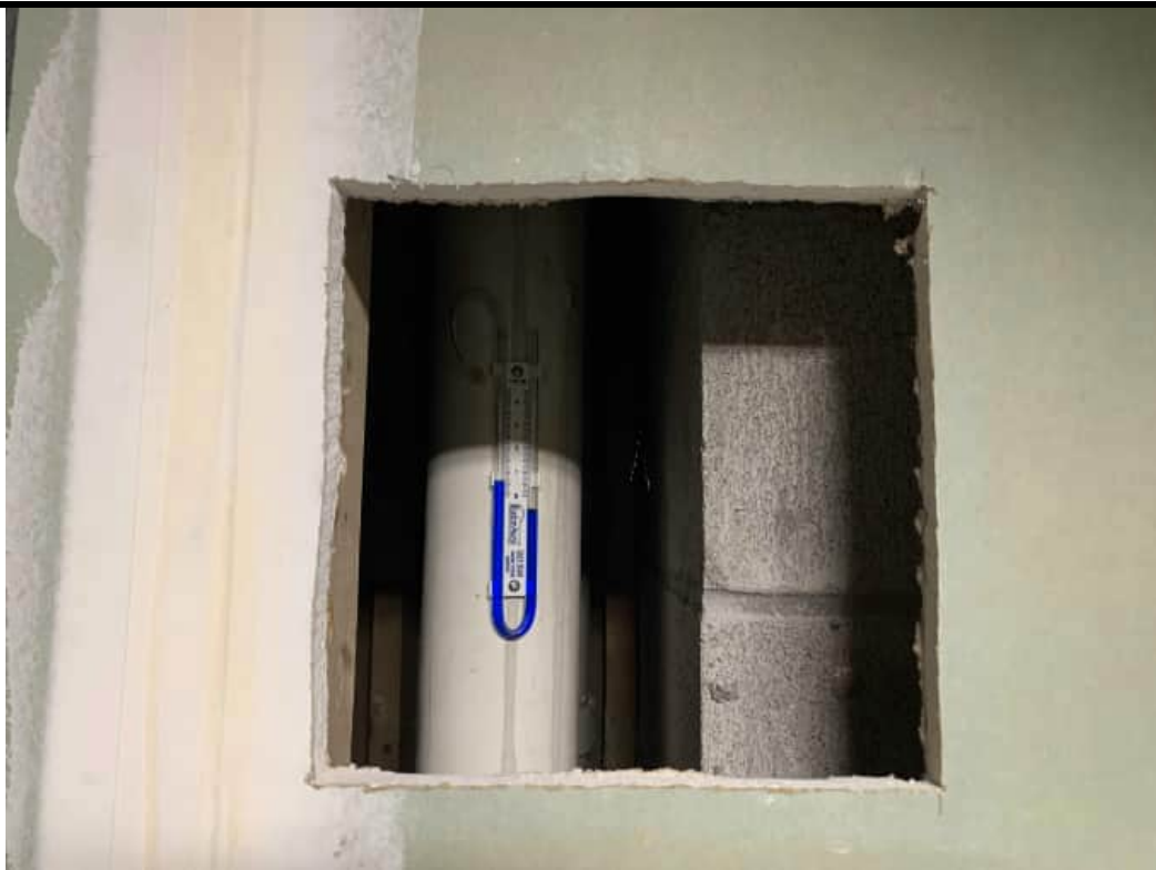
Photograph 19. View of manometer and vertical riser pipe for SSDS at 140 State Street (access via basement level) (12/20/24).
