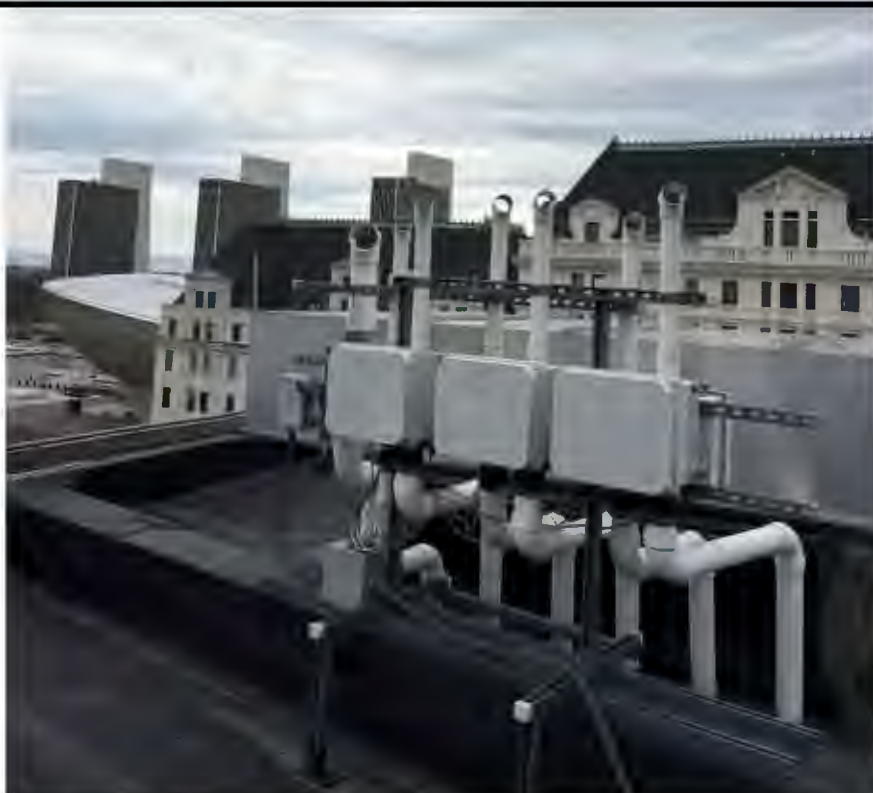
Photograph 3. Roof-mounted fan units for individual sub-systems at 144 State Street (4/13/2026).
