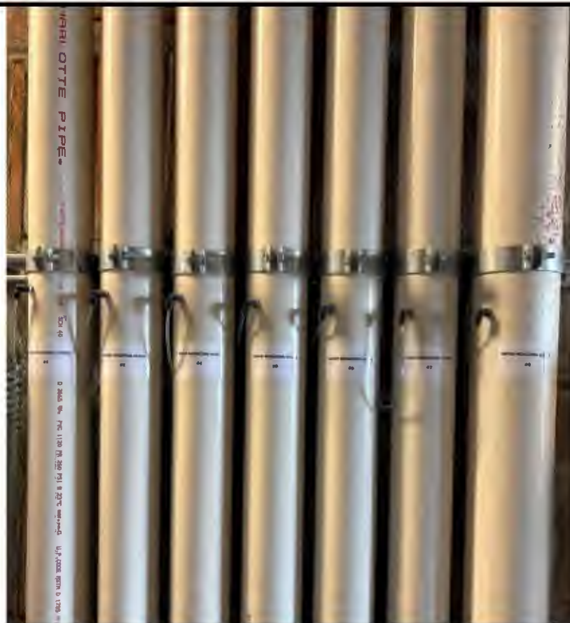
Photograph 1. Riser piping for the seven individual subsystems comprising the sub-slab depressurization system at 144 State Street (4/13/2026).
