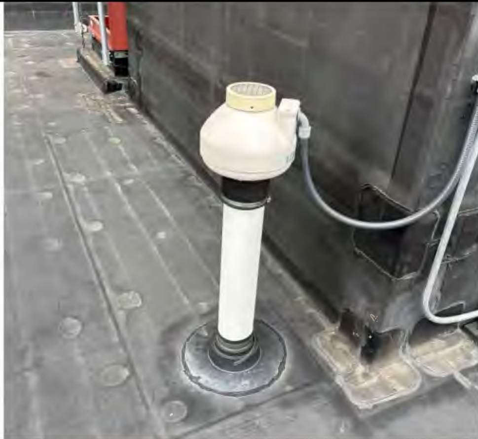
Photograph 13. Roof of 140 State Street building; exhaust stack, fan and switch for SSDS (4/13/26).
