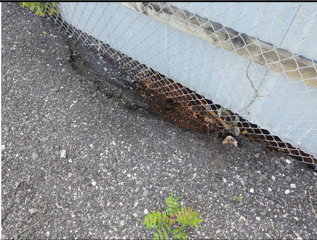
Photograph 5. RAP erosion from steam blowdown. See photograph 6 for condition post repair.
