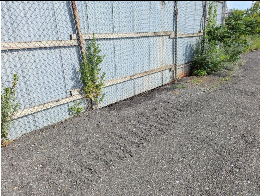
Photograph 6. RAP erosion from steam blowdown subsequently repaired by the APDC.
