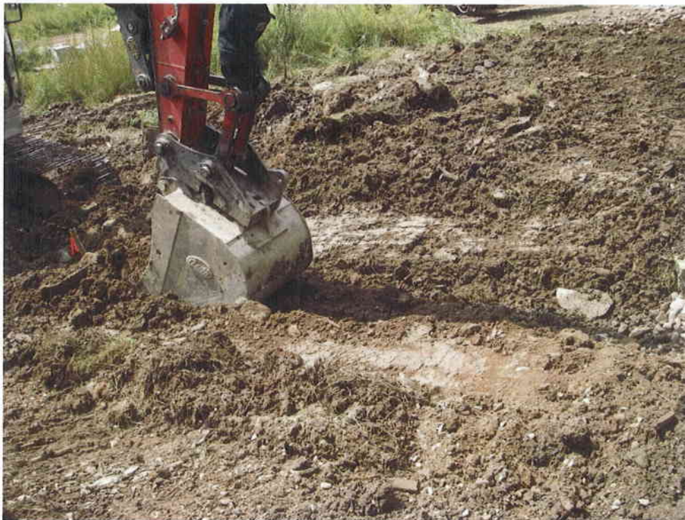
8. Step 2 of channel construction. Sub-grades were excavated for the streambed and bank treatments downstream to the location of the next grade control structure to be built. Rough grades were dug with the excavator and fine-tuned by hand.
