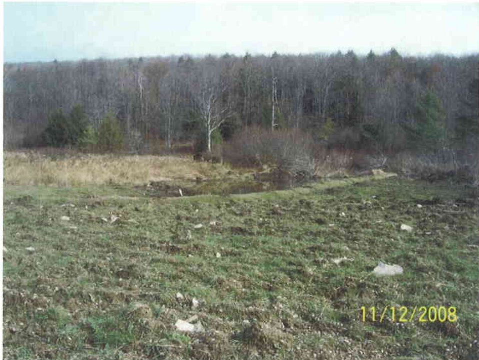
25. Level spreaders were constructed to maintain the hydrology needed to sustain existing wetlands adjacent to those areas disturbed during construction of the stream channel. Restored wetland areas were treated with peat and seeded with a wetland seed mix.
