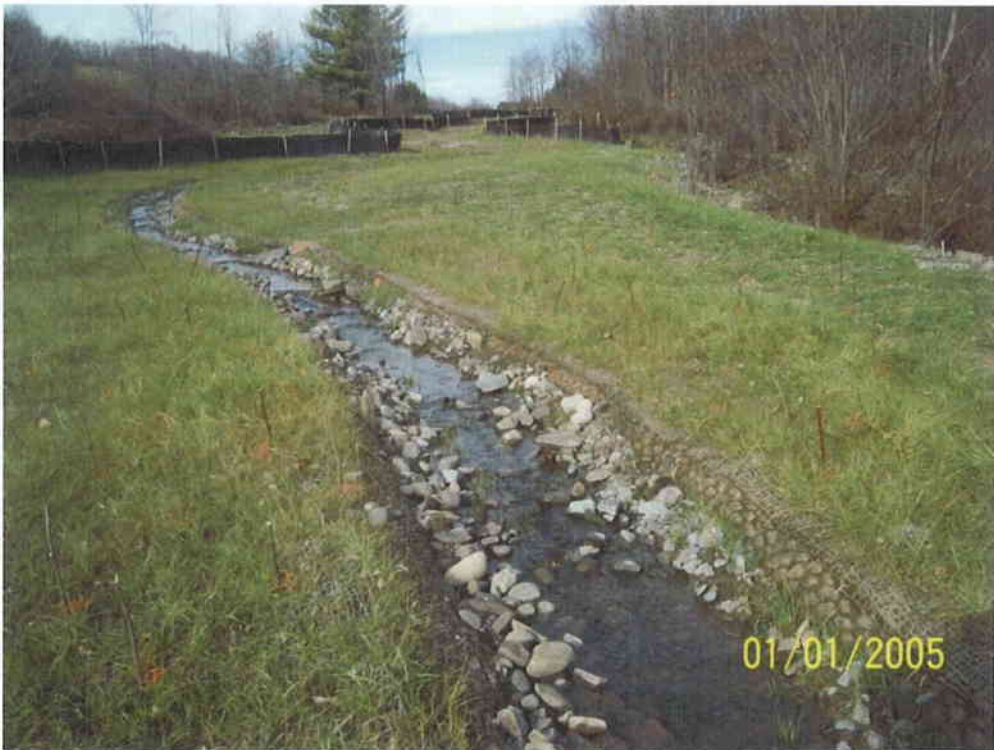
2. Post-construction view of stream Segment I. Restored channel has ample floodplain access, appropriately sized bed material, and stable channel geometry based upon reference reach conditions.
