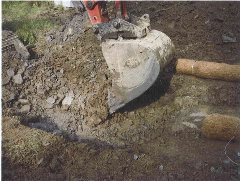
11. Step 5 - A footer was excavated at the location of each cross-vane and log vane as indicated in the design plans.
