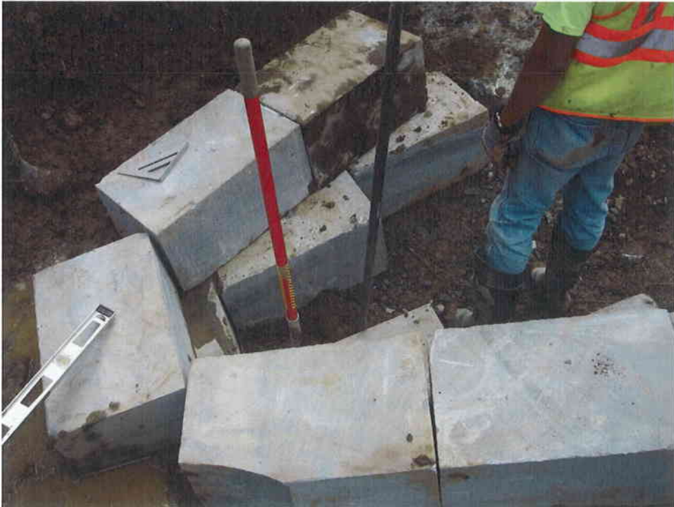
16. Step 10 - Vane rocks were installed. Vane rocks are set back upon the footer rocks to prevent undercutting of the structure.
