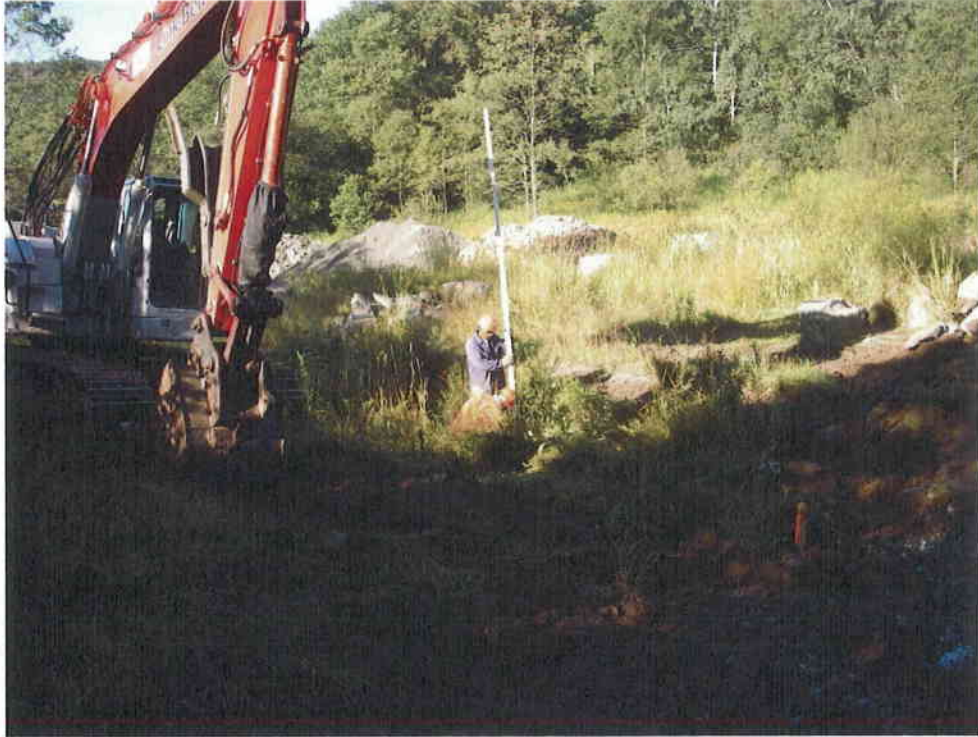
9. Step 3 - elevations of all sub-grades and structure footers were verified prior to continuation of the construction process.
