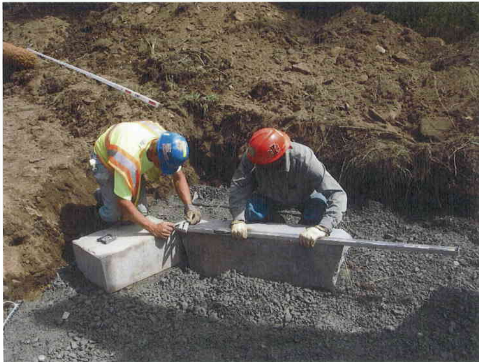
14. Step 8 - Footer rocks were checked to ensure proper elevation, arm slope and arm angle was achieved prior to installing the vane (upper) tier of rocks.
