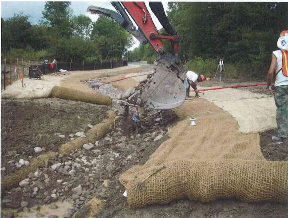
20. Step 14 - Imported gravel material was mixed on-site and placed in the stream channel. Over time, response of the stream to flood events will progressively sort and distribute bed material in an appropriate manner.
