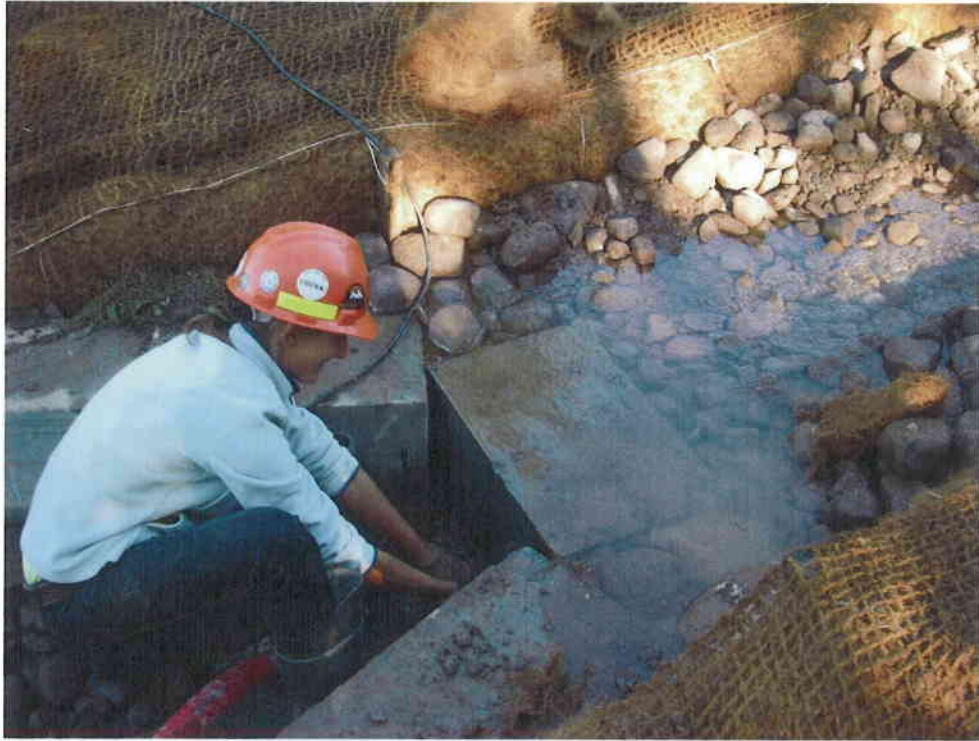
7. Step 1 of channel construction. Pump-around system was installed in a sump left at the end of the previous day's work, typically at a cross-vane structure. The entire downstream area to be constructed each day was dewatered.
