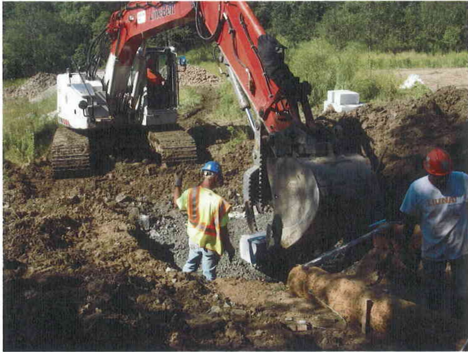
13. Step 7 - Rocks used to construct cross vanes were installed with an excavator, and fine-tuned in place by hand. Use of a hydraulic thumb is paramount to successful cross vane construction.
