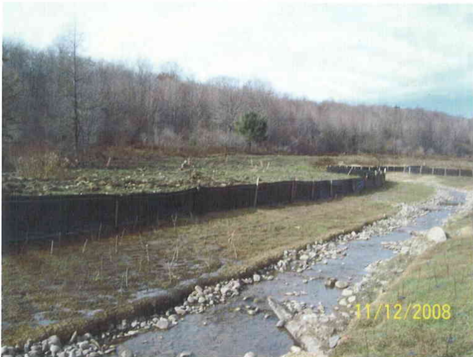
24. Live stakes were installed in the riparian corridor along the entire course of the restored channel.
