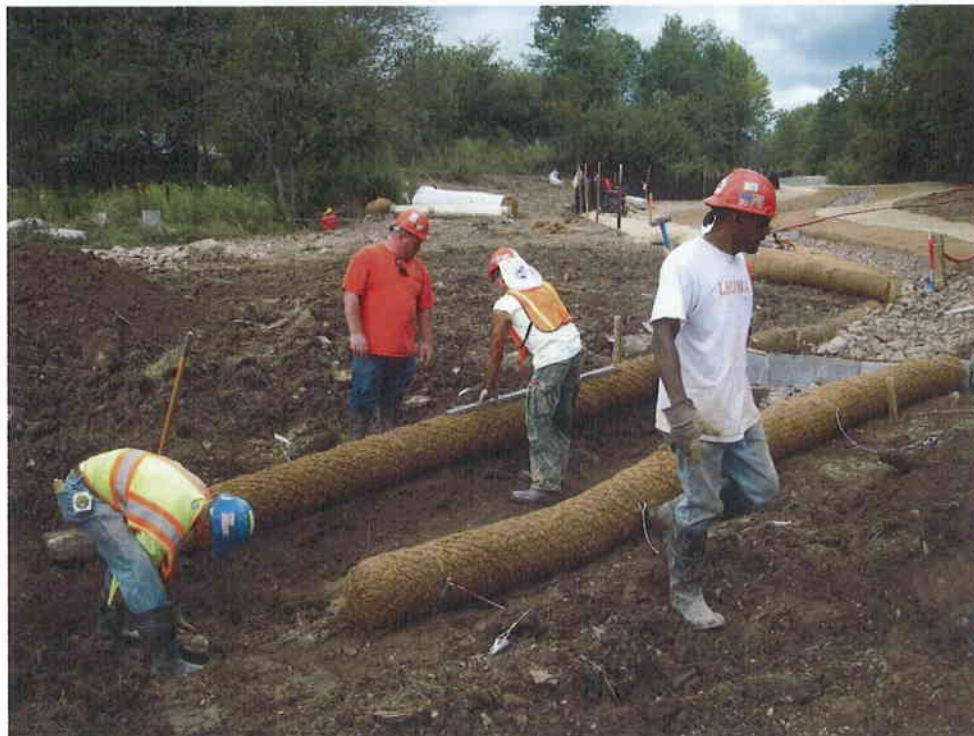
18. Step 12 - Streambank treatments were installed up to and beyond the location of the completed cross vane. Coir logs were used along the stream banks, with coir mats and erosion control fabric installed across disturbed portions of the floodplain.
