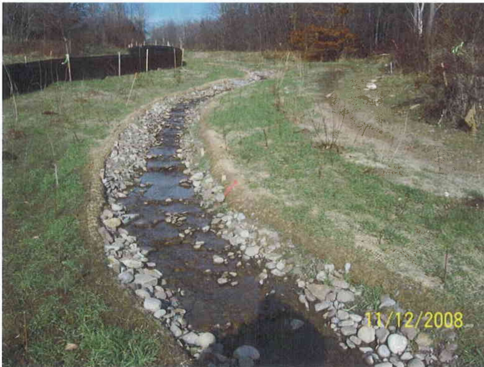
4. Post-construction view of stream Segment II. Channel has ample floodplain access, and channel sinuosity has been restored to reflect stable reference reach conditions.
