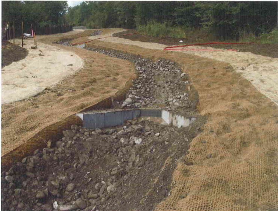
21. Step 15 - At the end of each work day, the pump-around system was disabled, and flow returned to the constructed channel. A sump hole was left at the downstream end of the last constructed cross vane to set the pump-around the following day.
