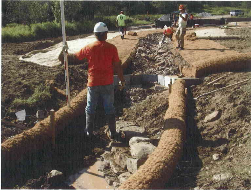
19. Step 13 - Finished stream bank and structure elevations were verified in the field prior to proceeding with the construction sequence.
