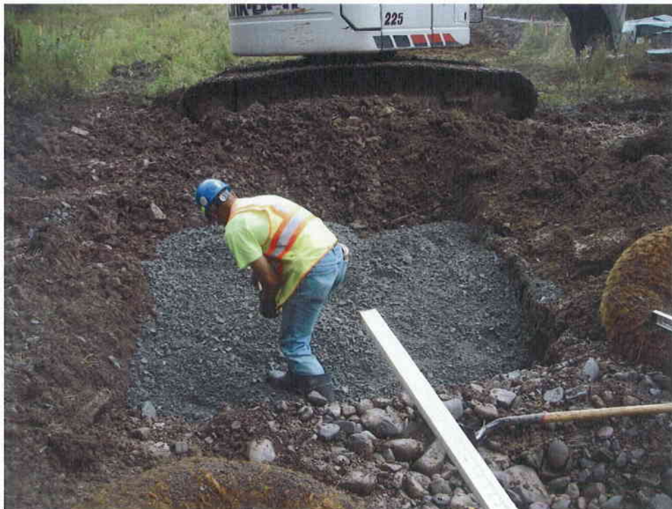
12. Step 6 - Gravel was placed to create a stable sub-grade for the placement of cross vane footer rocks. Gravel sub-grade was sloped so that footer and vane rocks would achieve the desired arm slope of 4% to 7% as indicated in the cross vane details and specifications.
