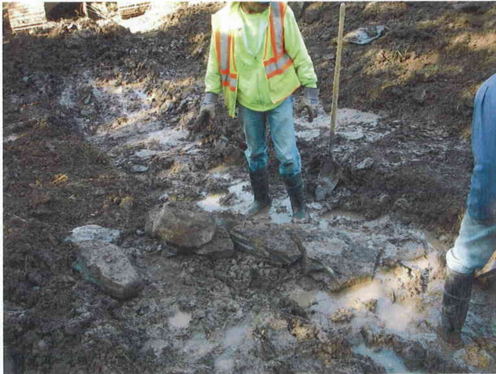
10. Step 4 - rock cascades were constructed by hand in locations indicated in the design. Sub-grade and final elevations were verified with survey equipment prior to continuation of the construction sequence.
