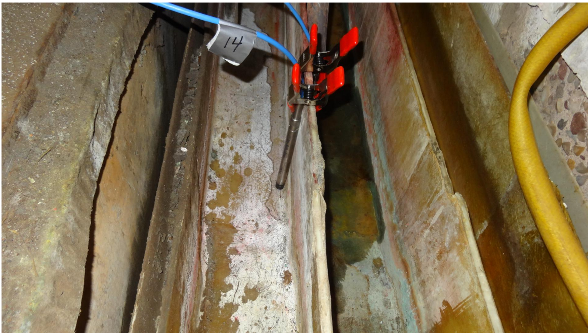
Photo 4 – Typical level sensor installation
