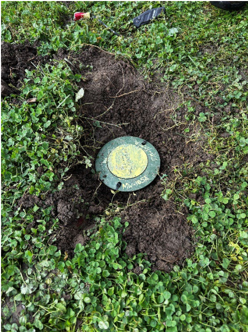
MW-105A covered with PVC cap
