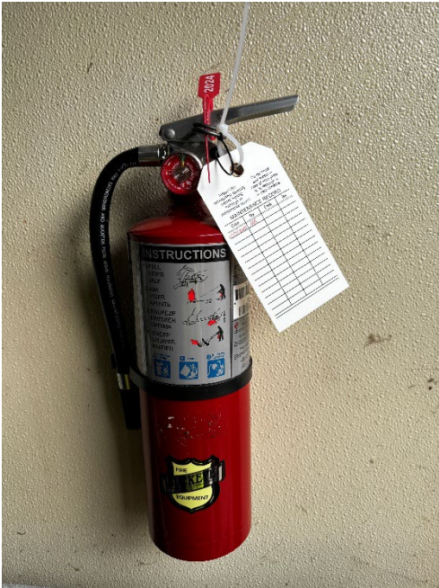
Fire Extinguisher @ Treatment Building
