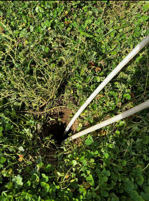
MW-105A over grown, found with no cover, no j-plug and excessive dirt, well was dug out and sampled for VOCs
