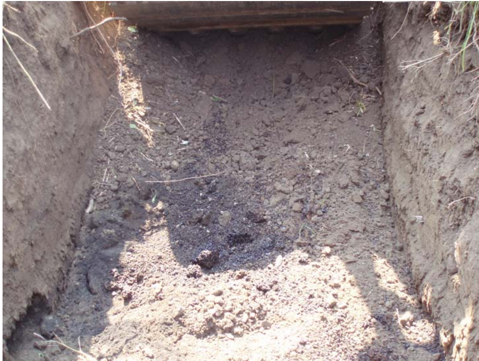
Photograph #11 – Facing west along TP-222b. Unidentified wet material resembling asphalt aggregate w/ no odor observed, potentially associated w/ pipe bedding from lines aligned north-south along Wynantskill Creek.
