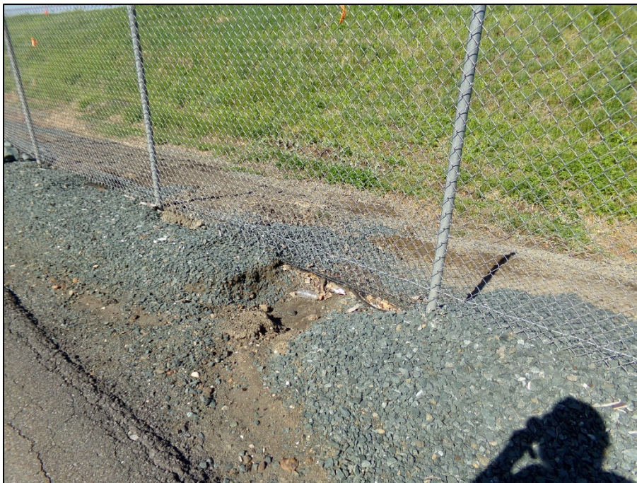
Washout of gravel beneath the fence prior to repairs.
