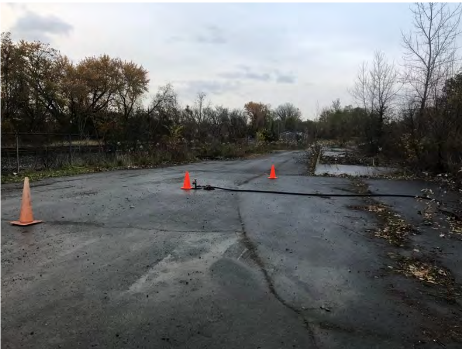
North side of property looking north. Minor cracks in asphalt visible.
