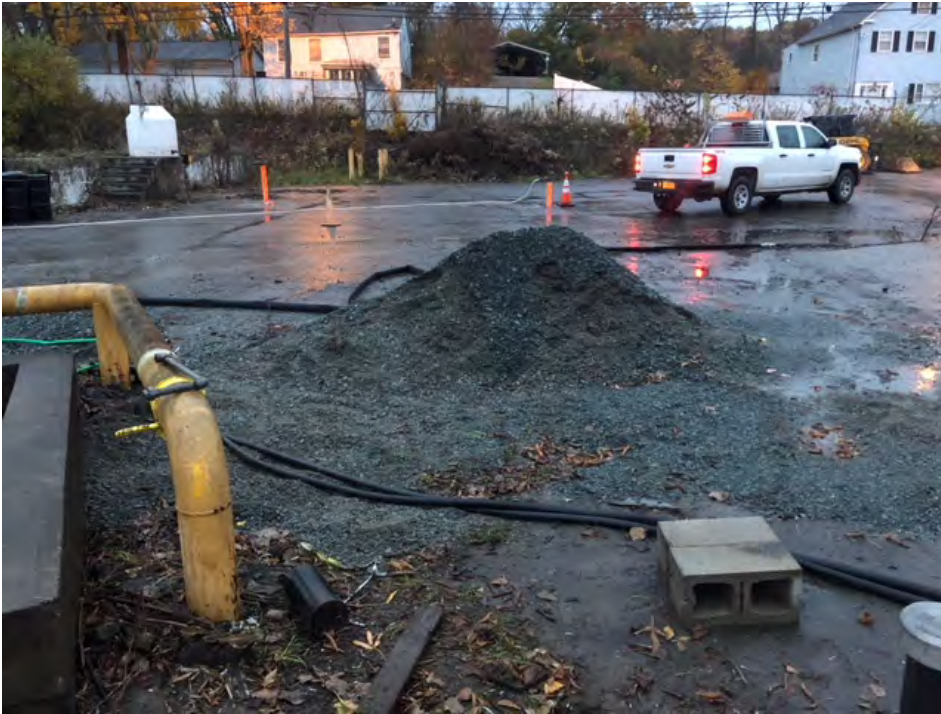
Cave in at culvert area near MW-B2 was filled in with gravel. Photo taken looking east.
