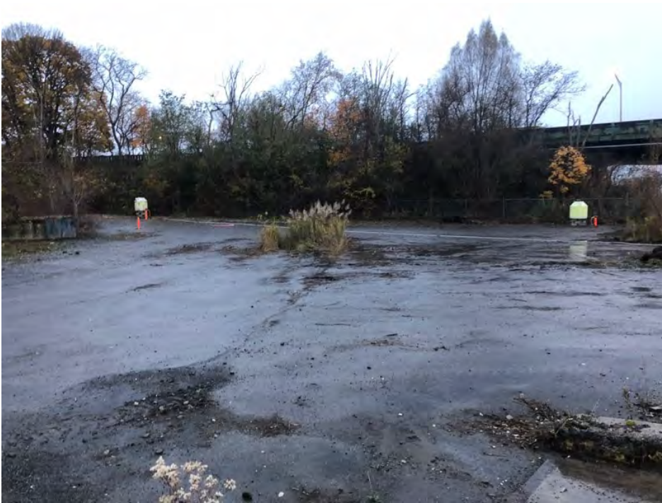
Onsite looking south toward newly installed wells. Minor cracks in asphalt and vegetation growing through asphalt visible in center of photo.
