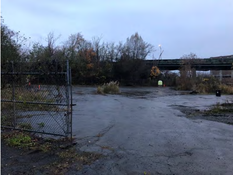
Offsite looking southwest through south entrance gate. Minor cracks in asphalt.
