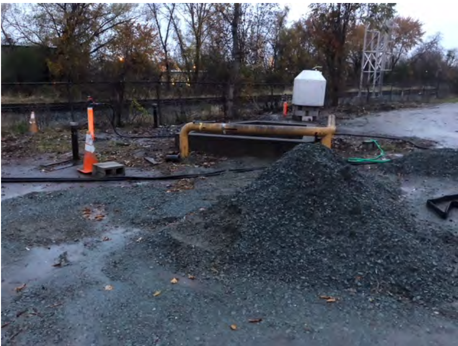
Cave in at culvert area near MW-B2 was filled in with gravel. Photo taken looking west.
