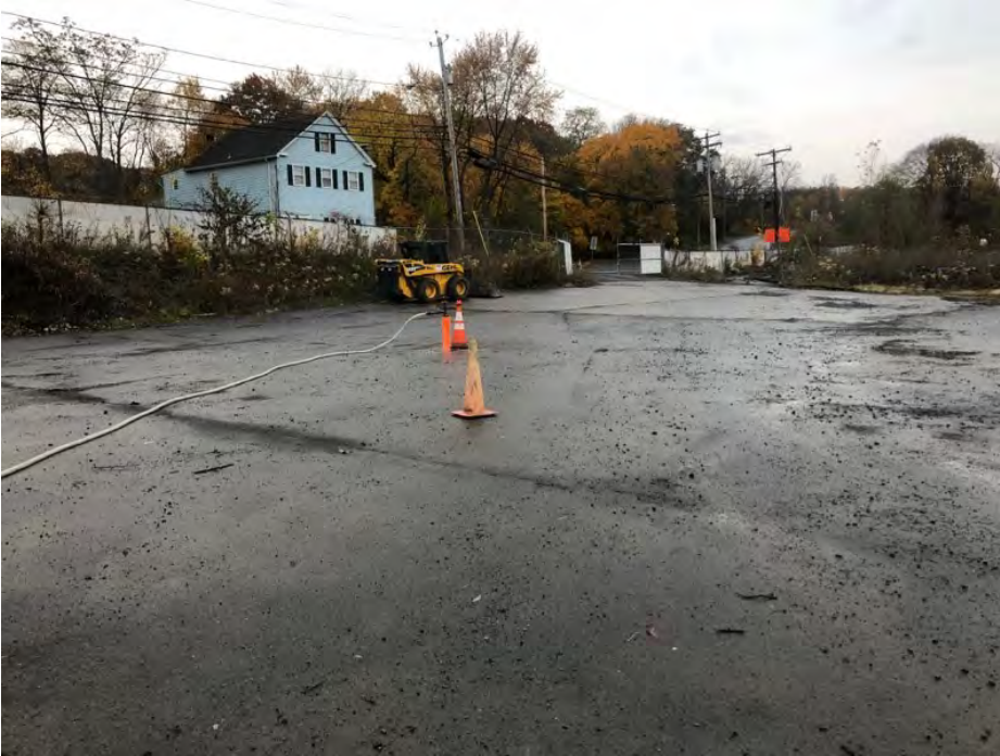
North side of property looking southeast toward north gate. Minor cracks in asphalt visible.
