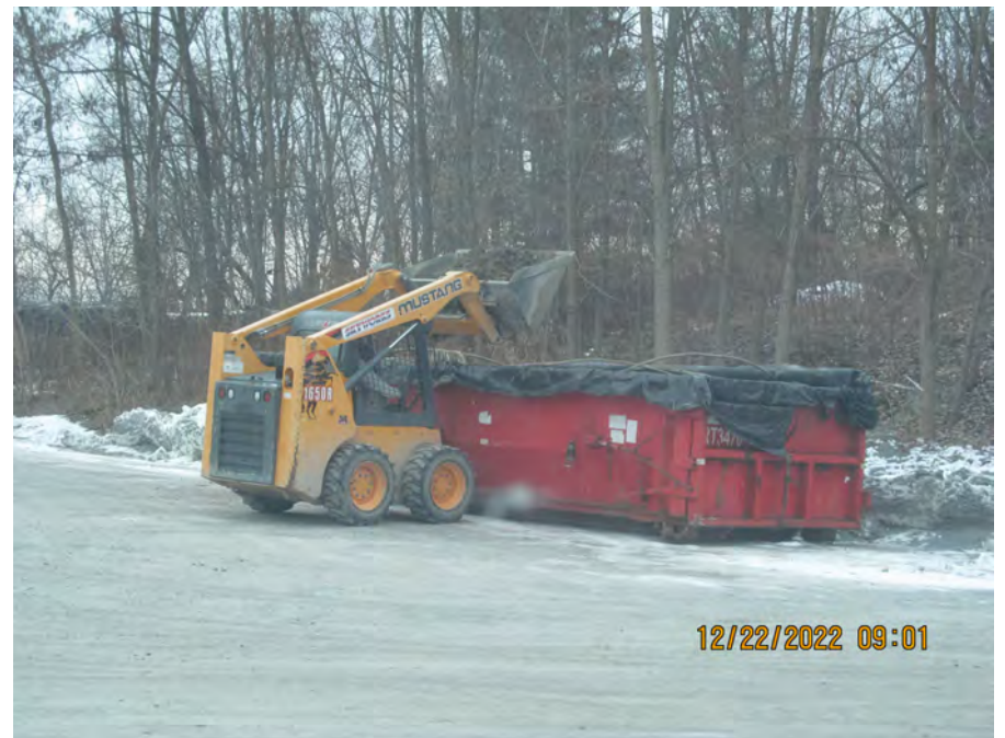
transfer material to rolloff 4
