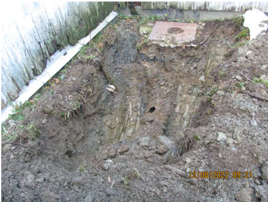
existng 12 inch CMP found
