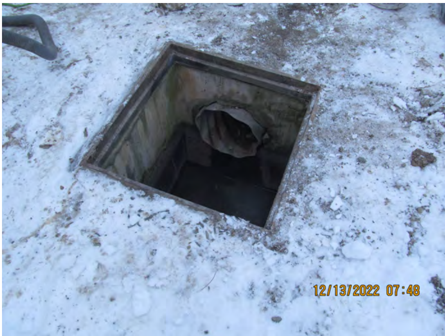
cb9 leak under culvert
