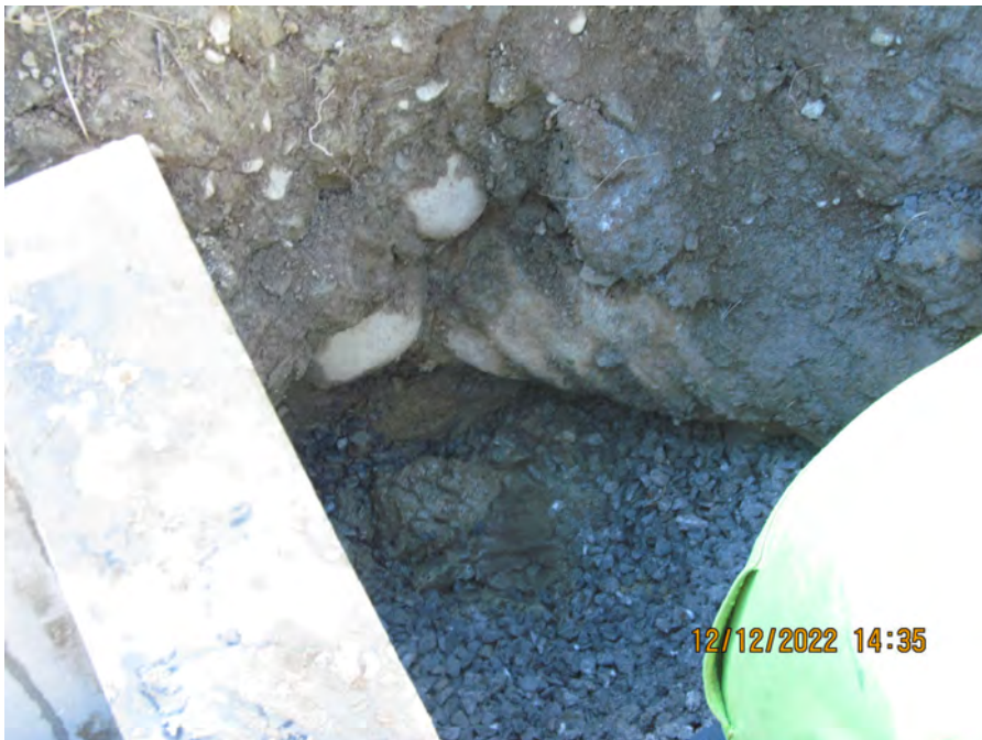
cb7 line plugged
