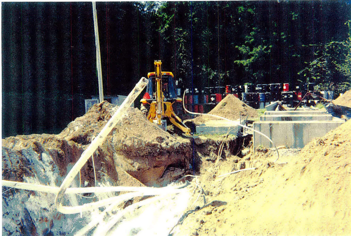
Photo 1: View looking towards pump house and Minebolt Resin Tank Cradles
