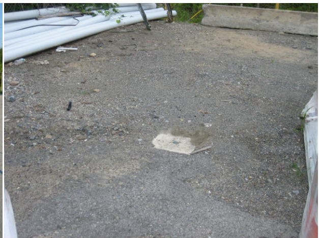
Monument #2 Intact But Damaged (Taken 9/2/13)
