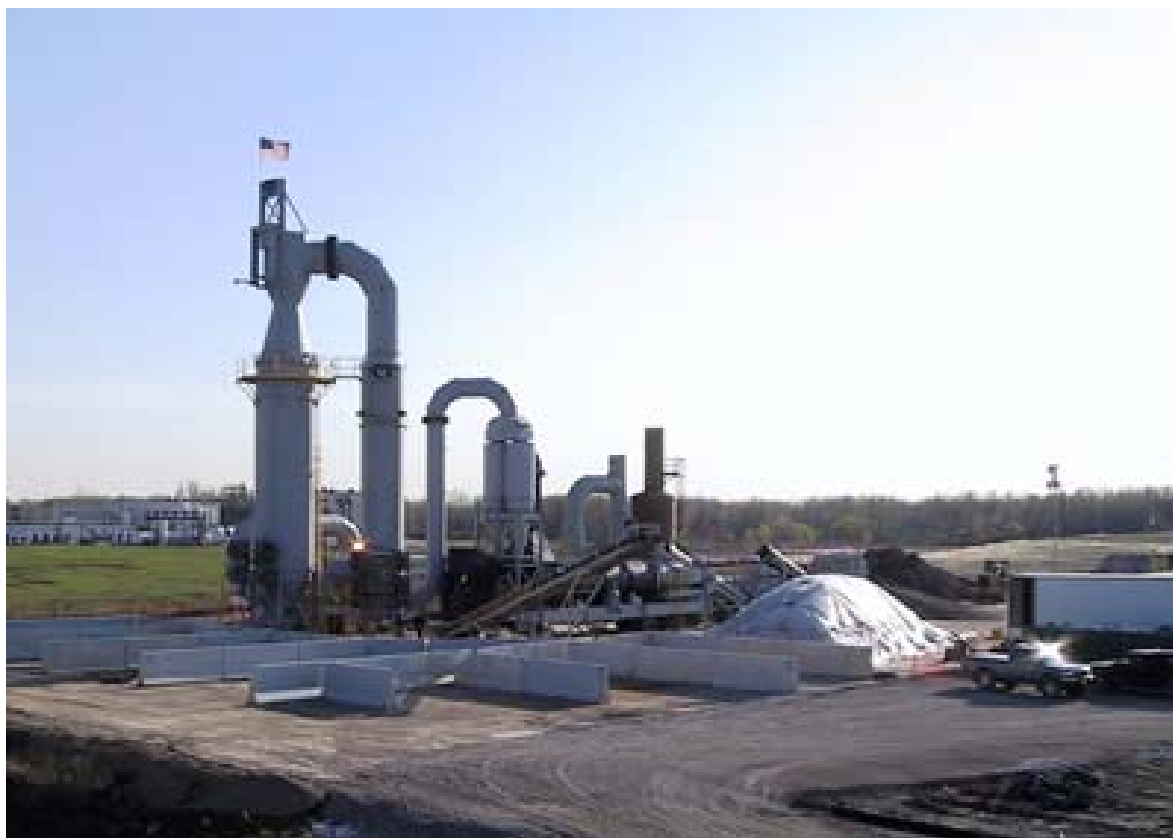
Figure 2.1 ESMI's Direct Heated Thermal Desorption Unit
