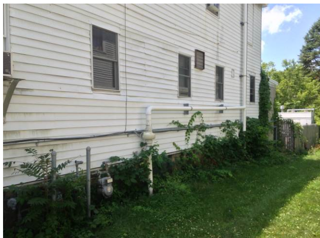
SSDS Blower and Piping
