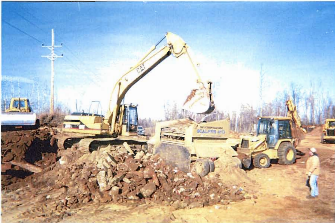
13. Stump Dump. Excavator, Loader, Shaker Screen and Bulldozer during excavation of Area 3
