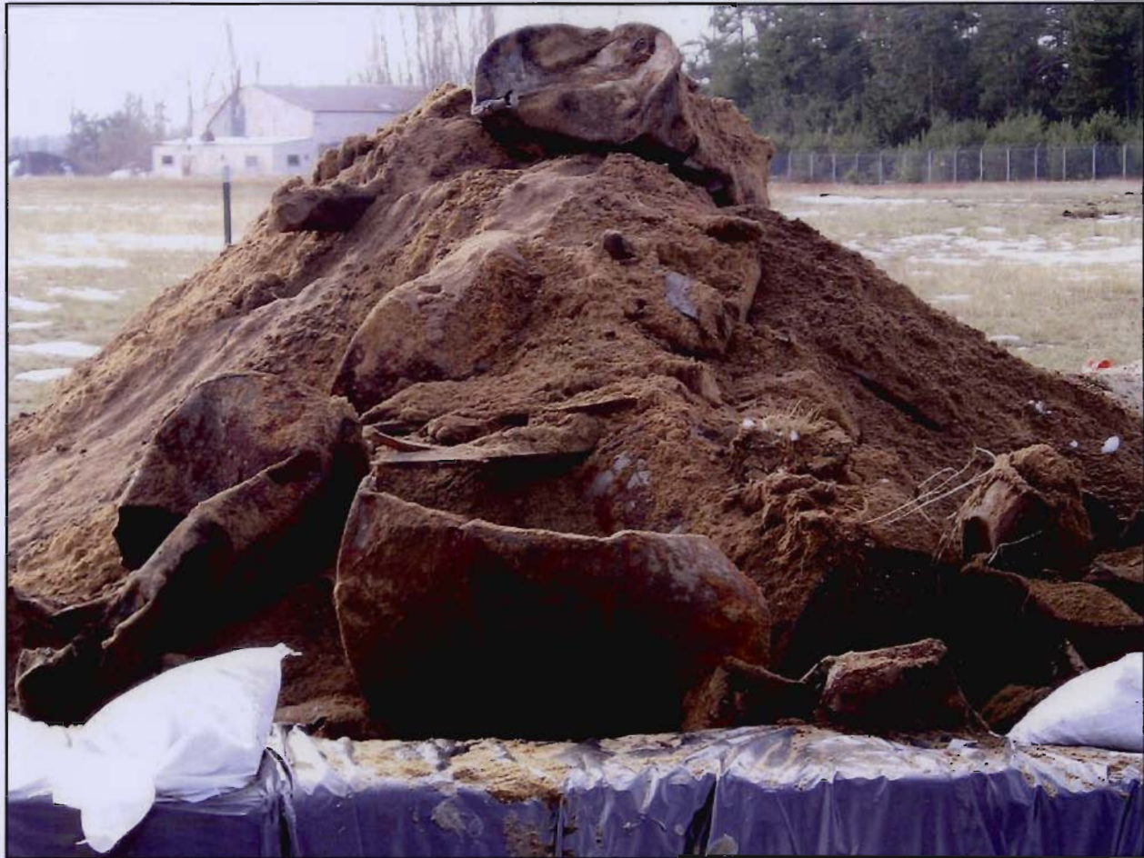
Photo 1 – Stockpiled soil and drums recovered during the initial drum and soil removal (17 NOV 2003)
