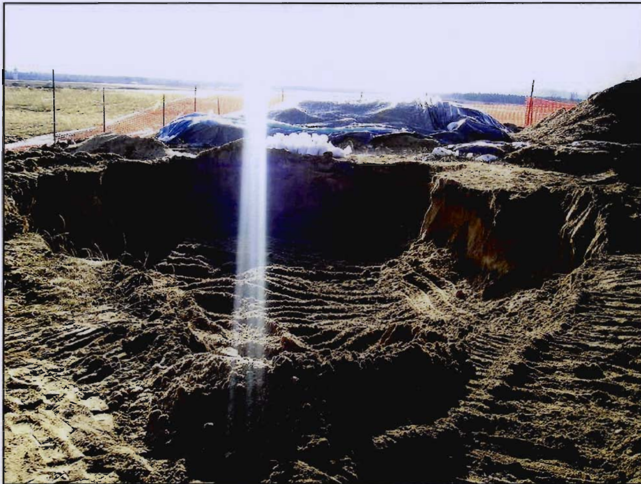
Photo 2 – Extent of excavation at conclusion of initial drum and soil removal (25 NOV 2003)
