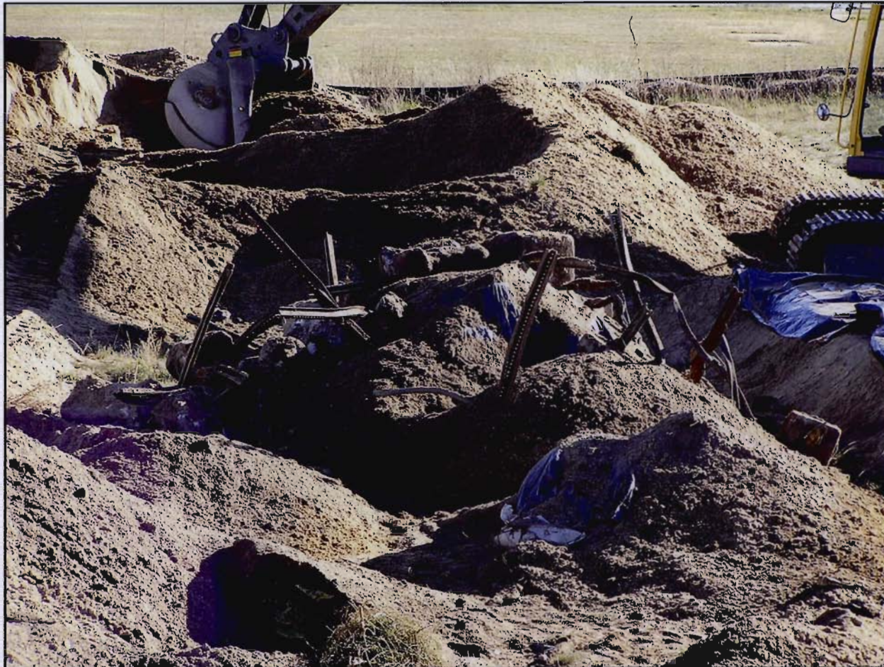
Photo 7 – Example of metallic debris recovered during third soil removal. Recovered debris included fence and sign posts with concrete, rail ties, rail, cable, and wire (13 OCT 2004).
