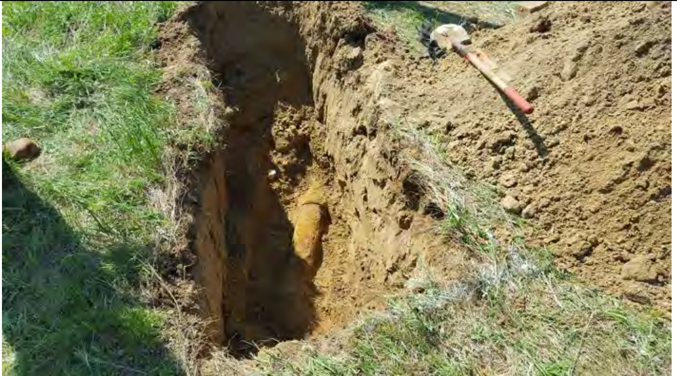
GPR detected the 8" metal pipe at a depth of 3' and we excavated that anomaly to examine the pipe.
