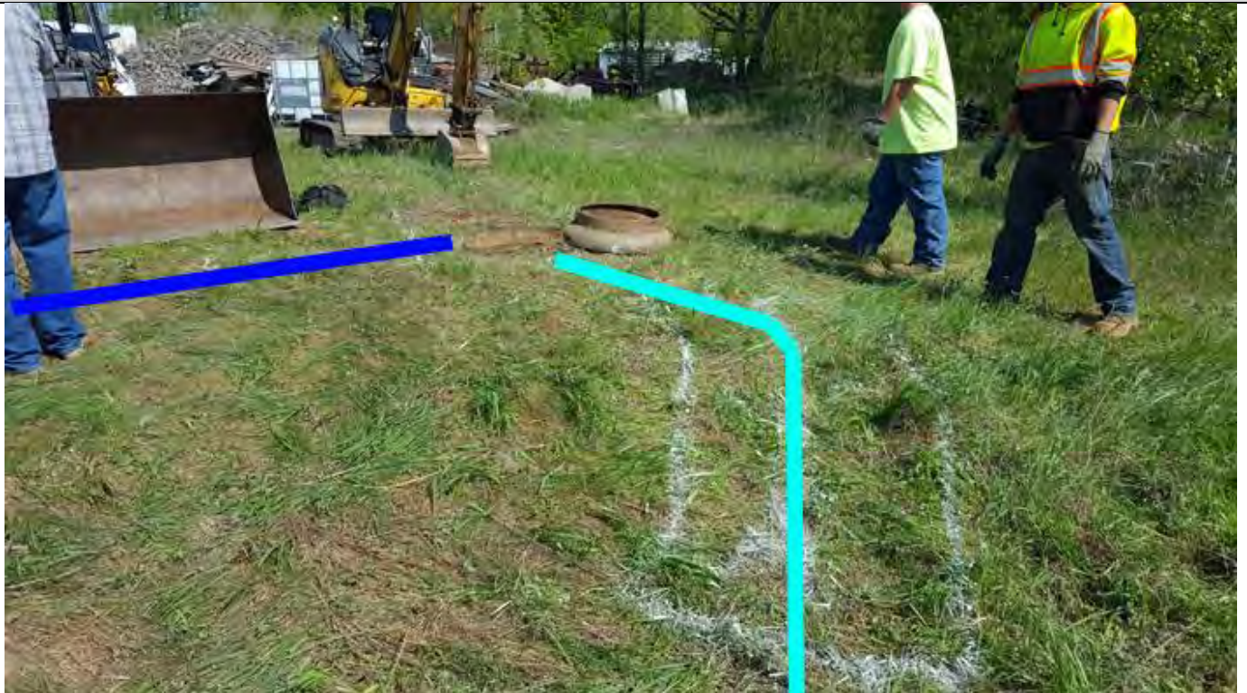
North facing view showing the manhole cover removed from the concrete vault. The light blue line is the trace of a metal pipe, while the dark blue line is the trace of a PVC pipe.
