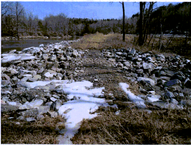
Picture # 5: View of inlet/outlet
