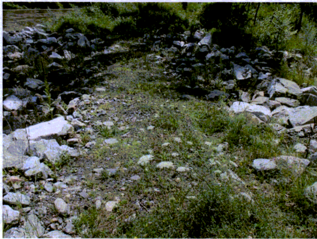
Picture # 5: View of inlet/outlet
