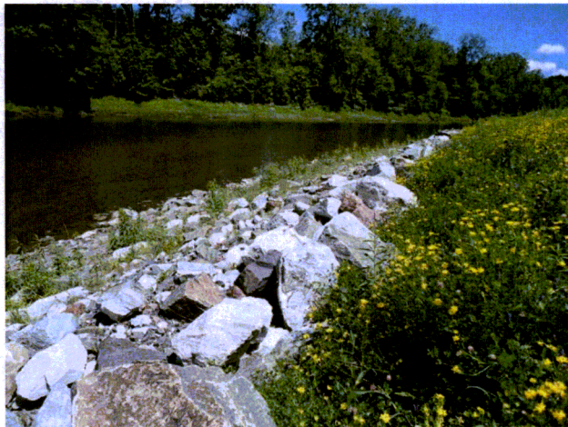
Picture # 2: View of deposition on riprap and growth on slope and in riprap
