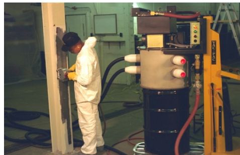
Worker is using the roto-peen (scabblers) attachment; VAC-PAC collection system shown with 55 gal drum.
