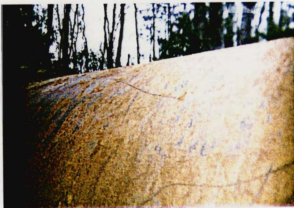
Photograph 30: Top of Tank 4 (6,000 gallon full oil tank).
