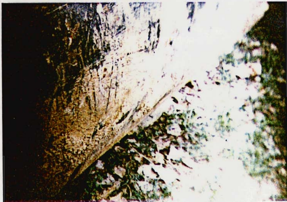
Photograph 27: Bottom of Tank 3, asphalt coating still visible.
