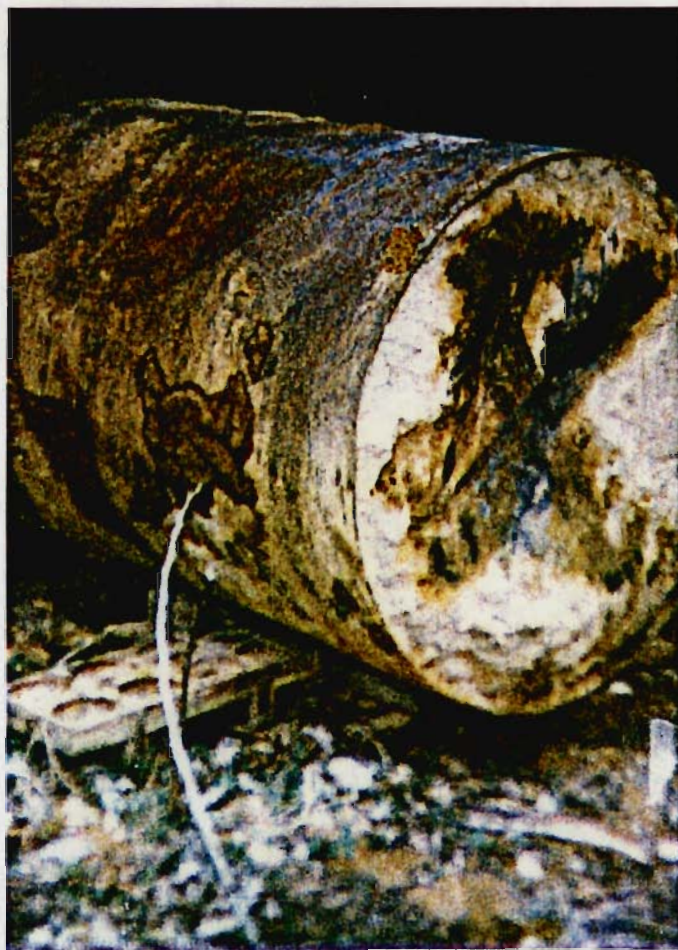
Photograph 25: Tank 2 (5,000 gallon gasoline tank).
