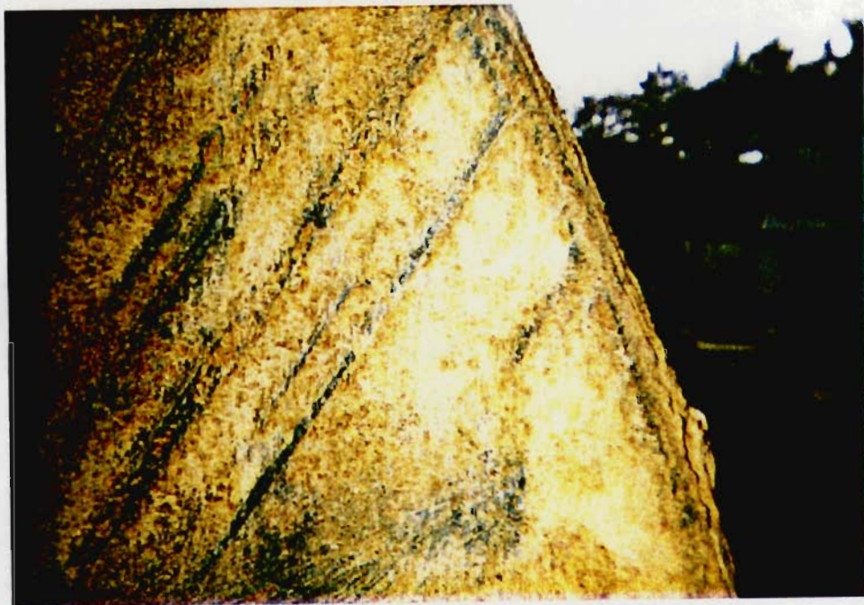
Photograph 28: Tank 5 (6,000 gallon fuel oil tank) seams with crane shovel gashes and surficial pitting visible.
