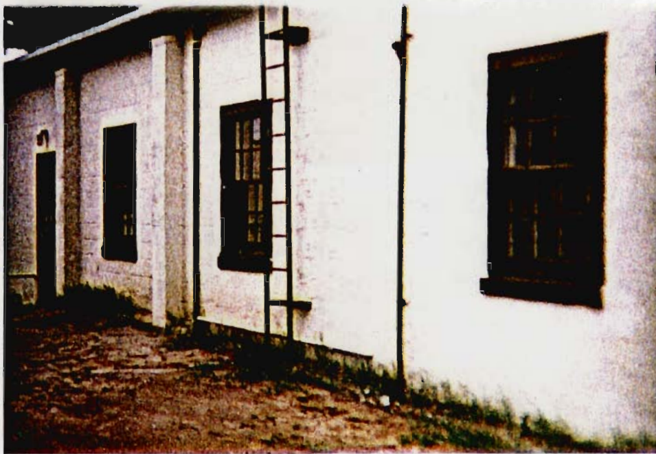
Photograph 7: Northwest wall of Building 15. Vent pipes for gasoline tanks (Tanks 1 and 2). Piping entered building below ground surface and through floor.
