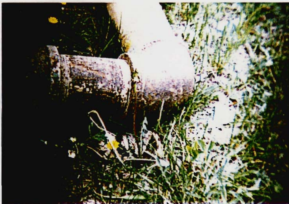
Photograph 32: Piping from Tank 4 and 5.
