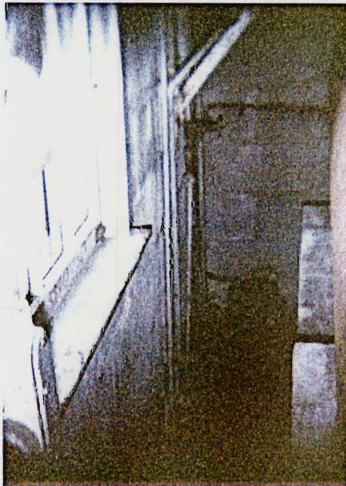
Photograph 8: Northwest interior wall of Building 15. Pipes leading from the two gasoline tanks.
